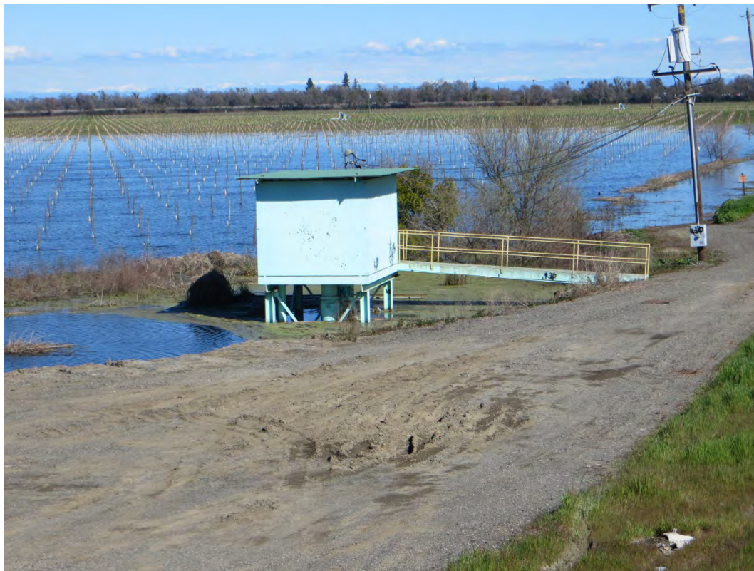
Figure 9. Existing RD 537 pump station
