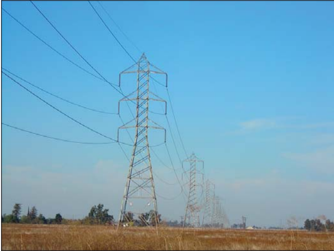
PHOTOGRAPH 1 – View to north from 16th Street and U Street; 230 kV powerlines.
