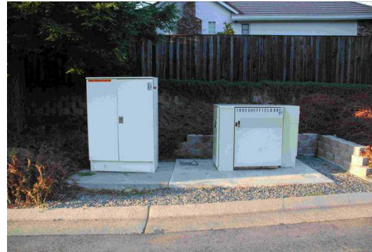
Figure 10 – SAI Box & Fiber Cabinet
