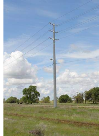
Figure 6 – 60 kV Double Circuit Transmission Line
