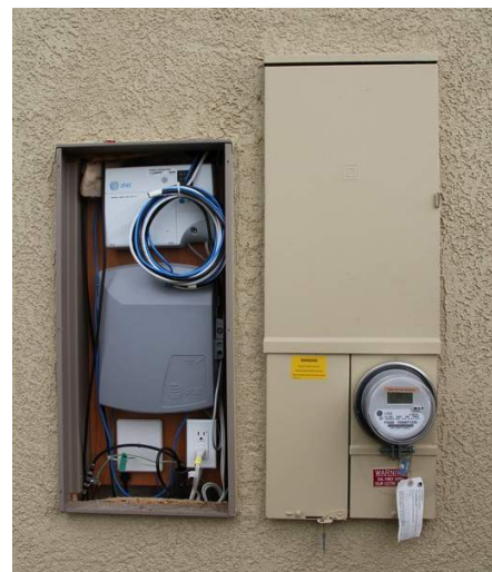
Figure 9 – ONT & Electric Meter Panel
