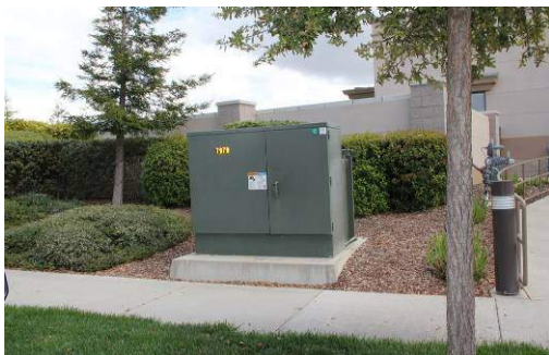
Figure 4 – Three Phase Transformer
