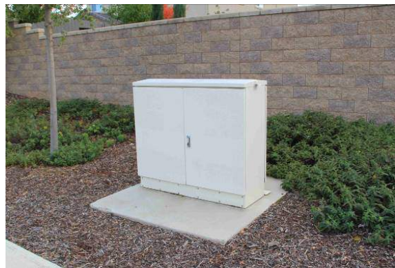
Figure 8 – AT&T Primary Flex Point
