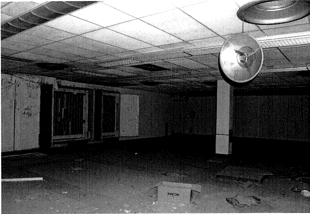
Plate 77: Control Center (Unit 61), Alpha Test Complex, 1956-1957. Interior of operations room. View of May 2005.
