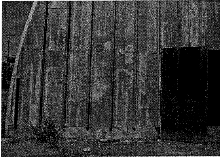
Plate 33: ASV Building (Unit 106), Solid Propellant Assembly Area, 1966. Detail of sheathing. Looking west. View of May 2005.
