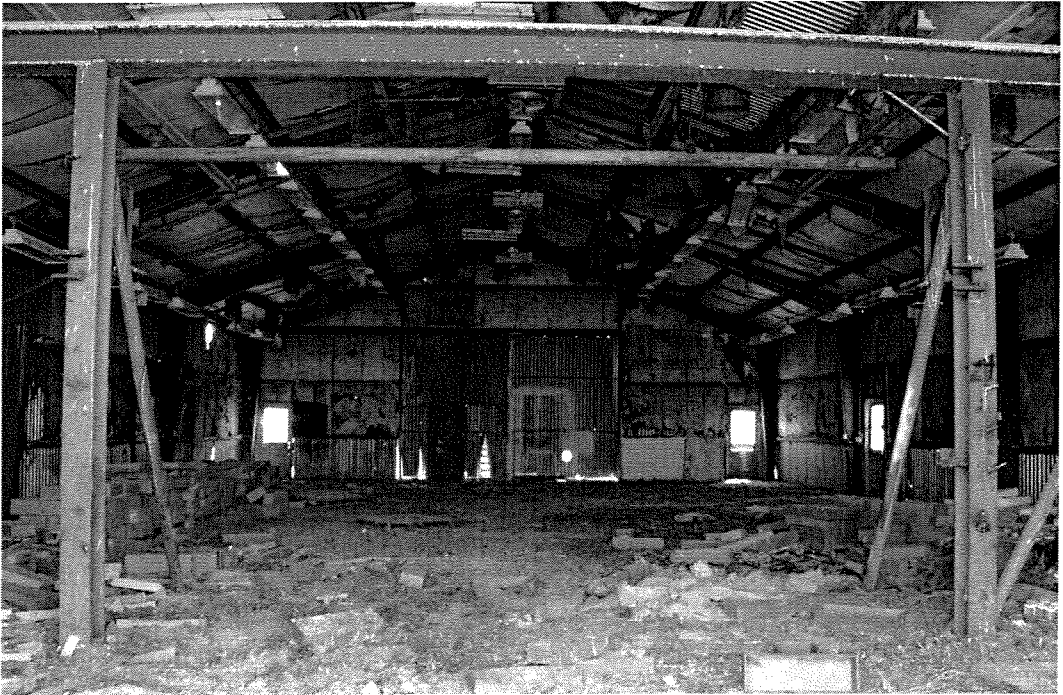
Plate 54: Assembly Building (Unit 93), interior, Sigma Test Area, 1956. Looking east. View of May 2005.
