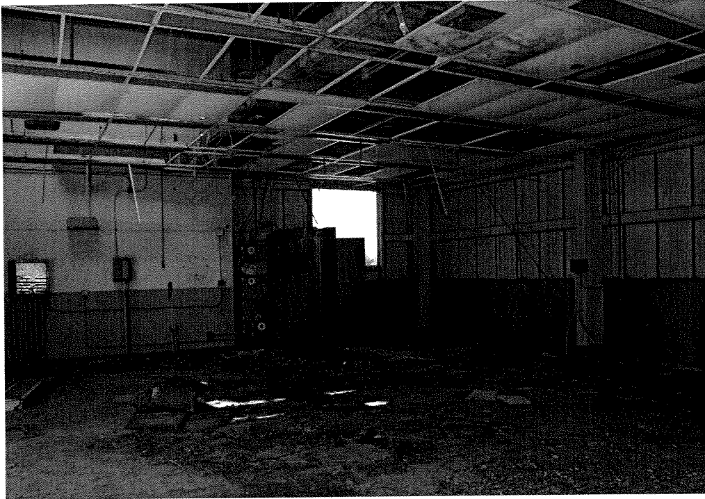
Plate 129: Beta Support Office No. 1 (Unit 142), Beta Test Complex, 1963-1964. Interior. Looking northeast. View of May 2005.
