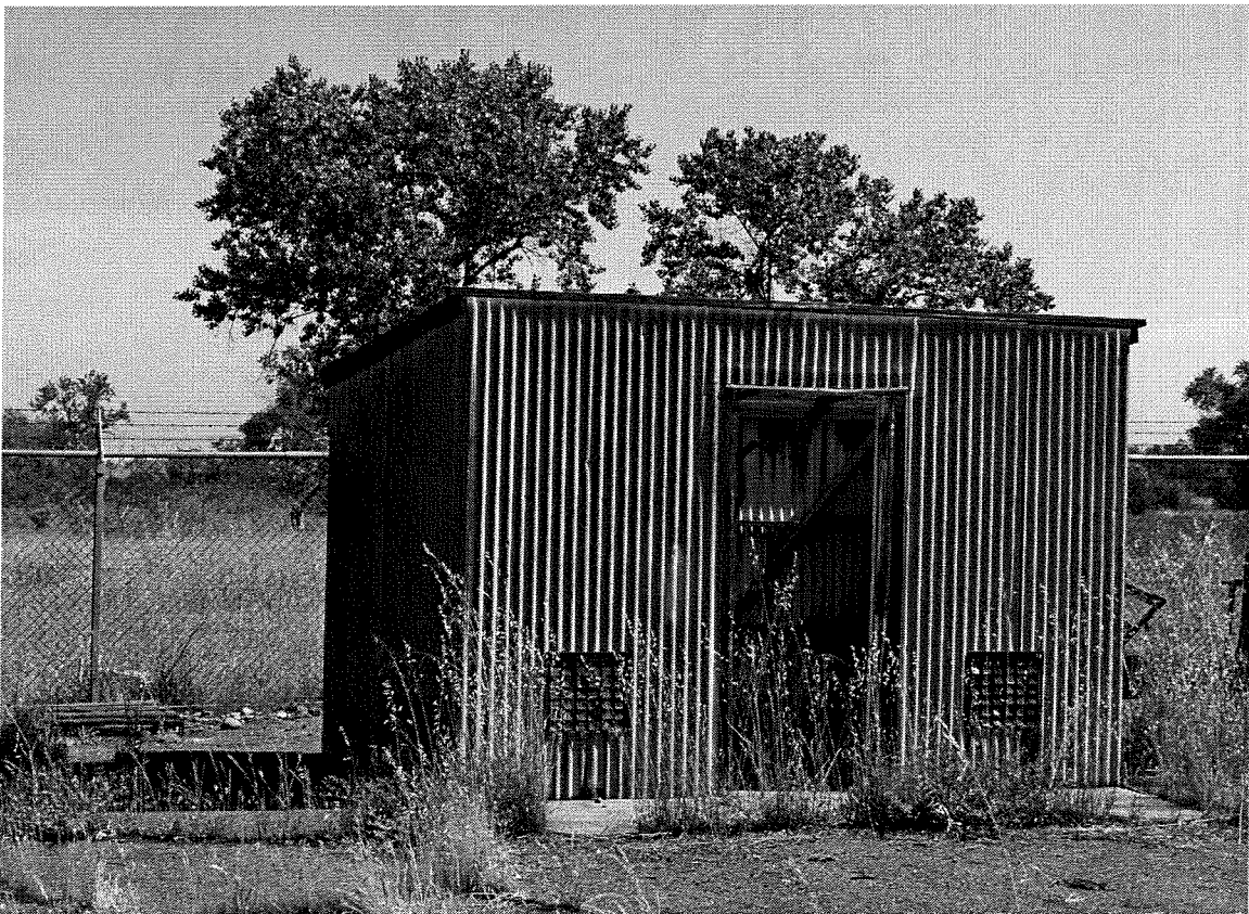
Plate 25: Paint Shed (Unit 109), located to the rear of the Assembly Building, Solid Propellant Assembly Area, 1956. Looking north/northeast. View of May 2005.
