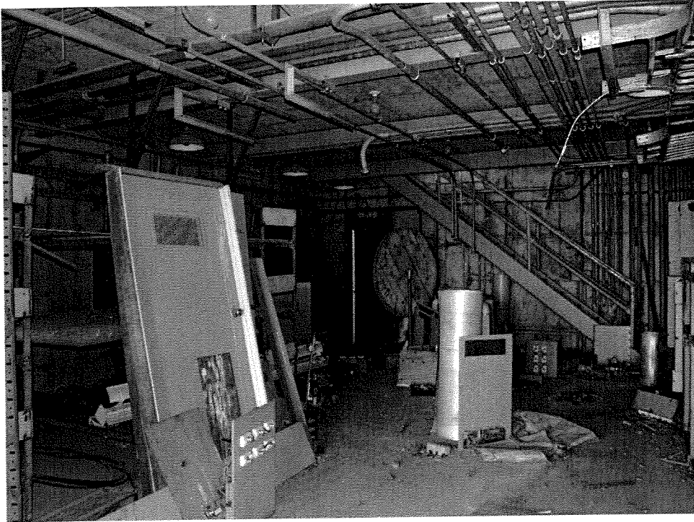
Plate 88: Test Stand No. 1, Alpha Test Complex, 1956-1957. Terminal room. Looking west/southwest. View of May 2005.
