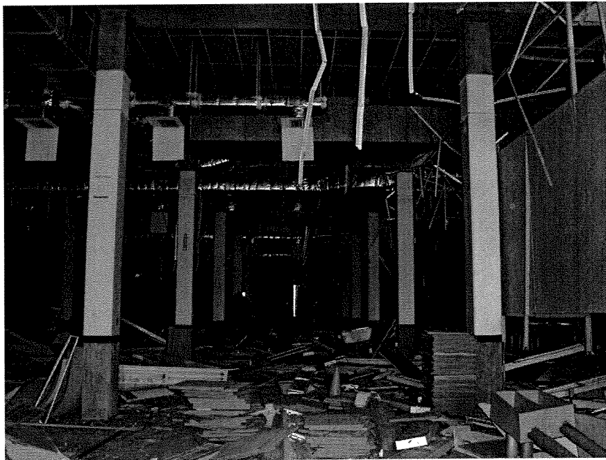
Plate 123: Test Control Center (Unit 121), Beta Test Complex, 1963-1964. Interior of main control room. Looking east/southeast. View of May 2005.
