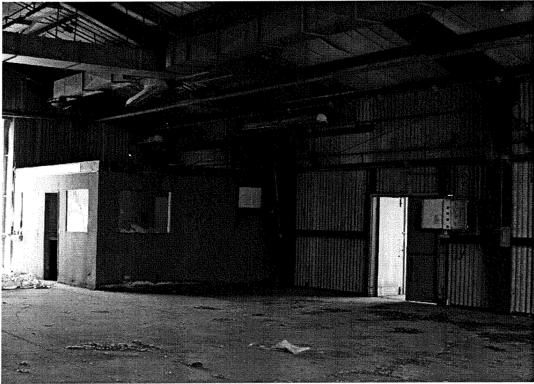
Plate 23: Assembly Building (Unit 103), Solid Propellant Assembly Area, 1956. Interior, looking southwest. View of May 2005.
