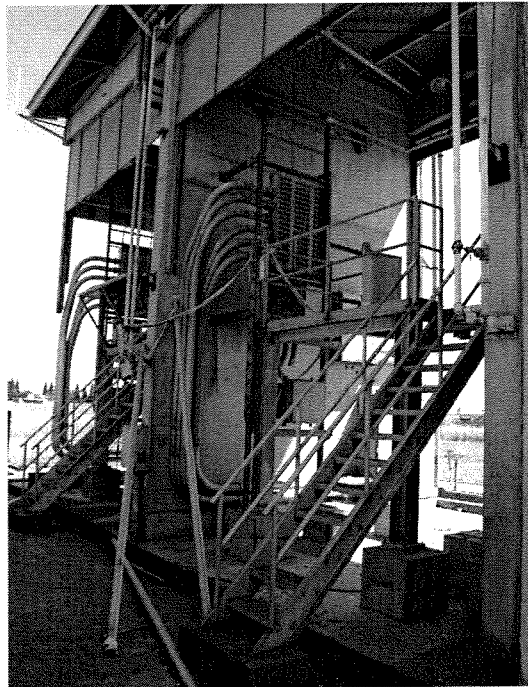
Plate 156: Test Structure (Unit 32), Gamma Test Area, 1964. Middle test cell, remnant. East test cell, background left. Looking northwest. View of May 2005.
