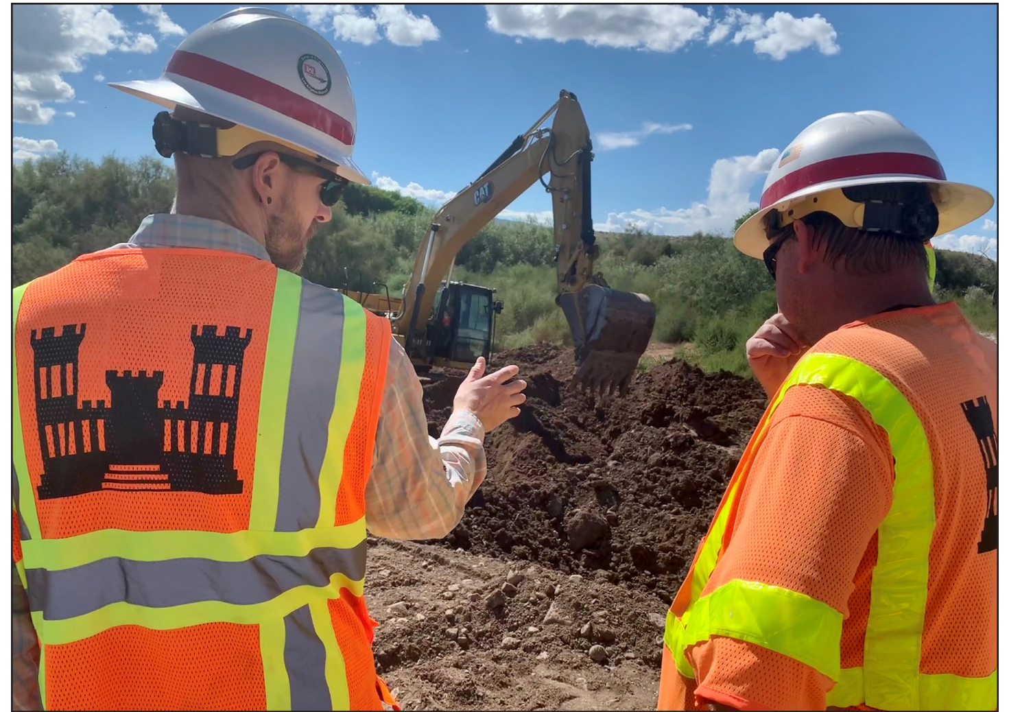
U.S. Army Corps of Engineers Los Angeles District Project Engineer David Silvertooth, left, and Quality Assurance Representative Clinton Griffin look out over a construction-reinforced embankment designed to protect critical infrastructure against flooding Oct. 5 in Duncan, Arizona. The embankment protects the town’s wastewater treatment station from similar flooding events.
