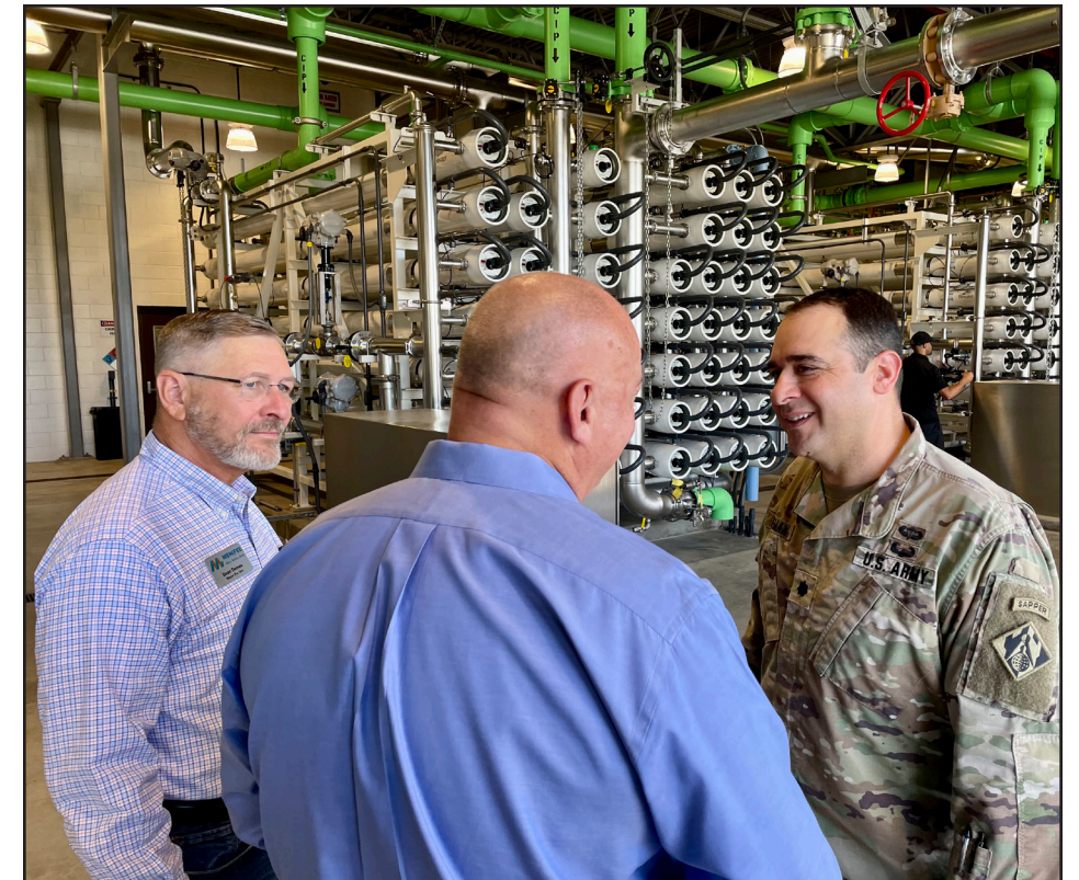
Lt. Col. Jeffrey Beeman, right, deputy commander of the Los Angeles District, talks with Menifee Mayor Bill Zimmerman, center, and Menifee Mayor Pro Tem Dean Deines during the June 23 grand opening of the Perris II Reverse Osmosis Treatment Facility in Menifee, California.
