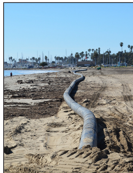
Pictured is a dredging pipe set down for emergency dredging operations Jan. 25 on the beach near Santa Barbara Harbor in Santa Barbara, California.
