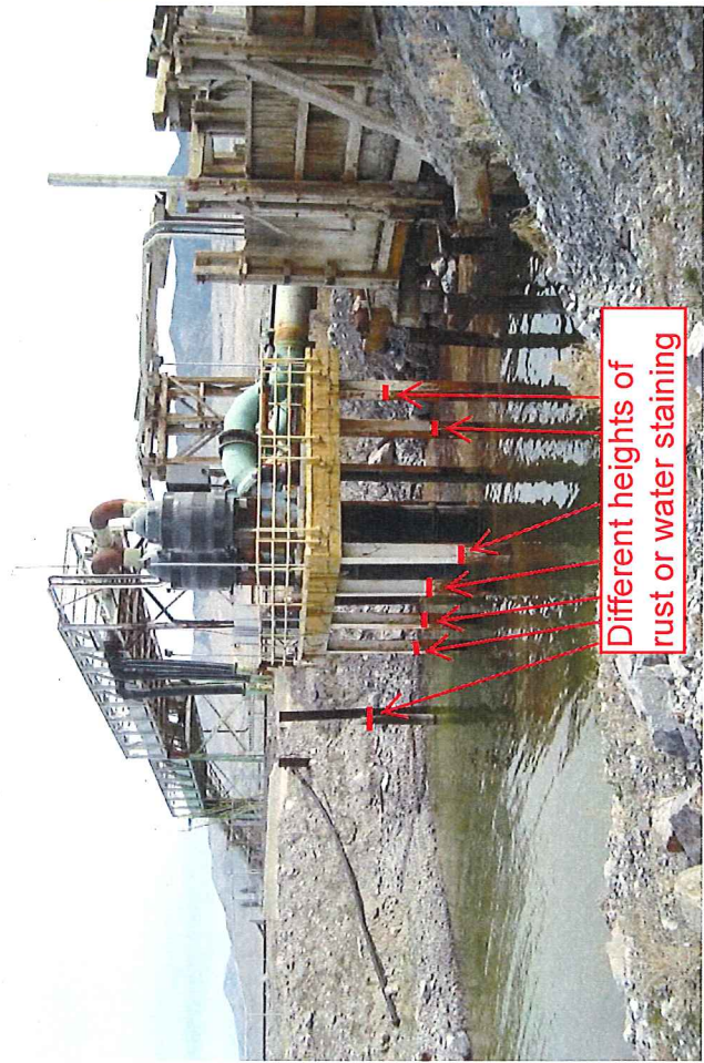
Uneven rusting of metal structures
