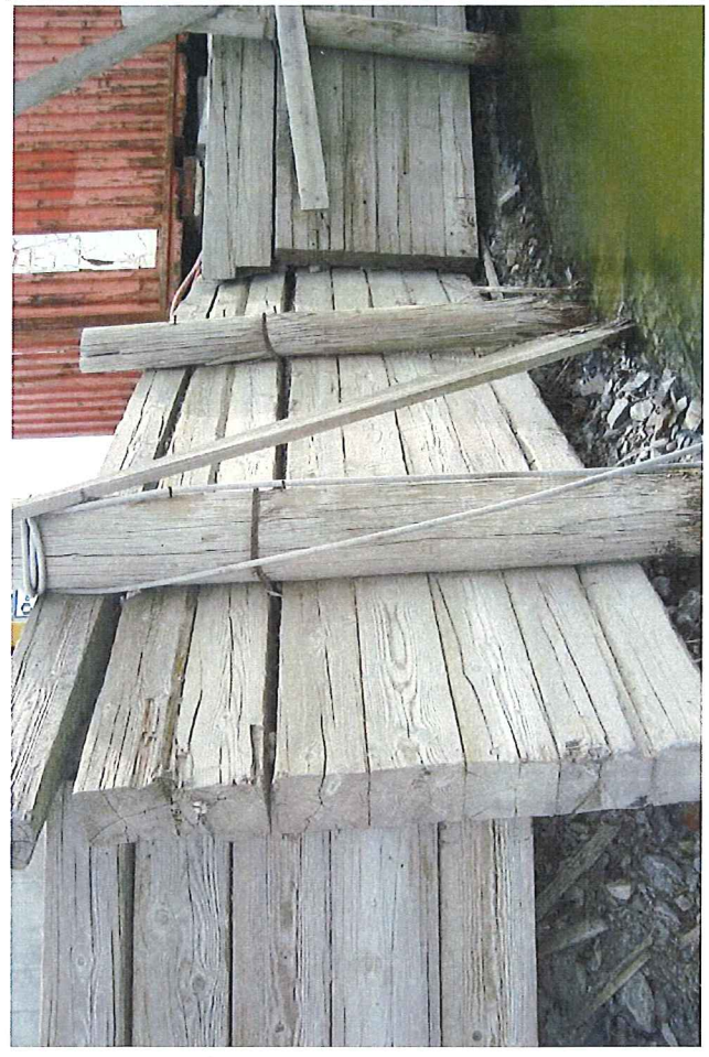
Water staining obscured due to bleaching effects of GSL's hyper-saline environment
