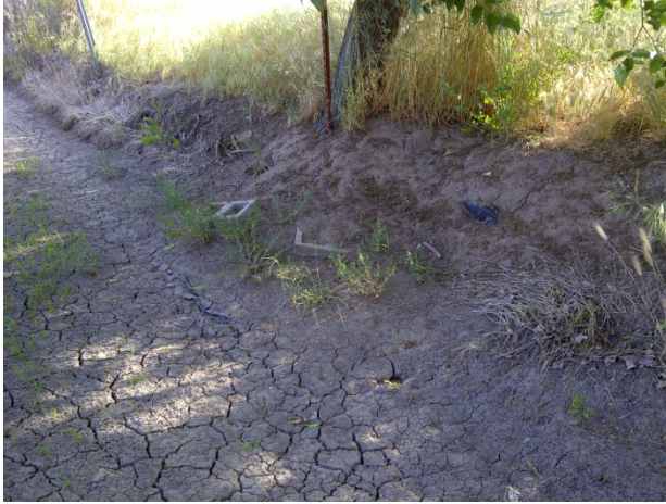
Photo 1 – The covered culvert connecting from the ditch to the pond. The very top of the plastic covering is visible in the photo.
