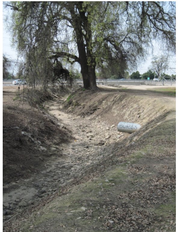
Outlet pipe for releasing water from dcCH17 to dCH3
