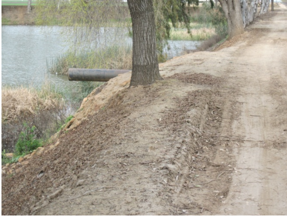
Outlet pipe for water pumped out of dCH19 to go into pb30
