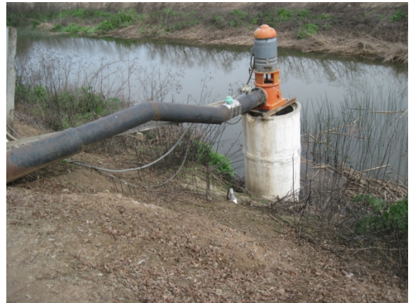
Close up of dCH19 pump
