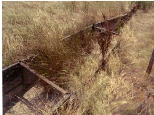
Photo 6. Close up of CH 1C where it exits the project site. The channel bed has been excavated and put in a flume to direct water flow through the adjacent property (June 2009).
