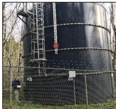
Robert Killey takes measurements of the SWB Tribe's water tower to better recommend any stabilizing options.
