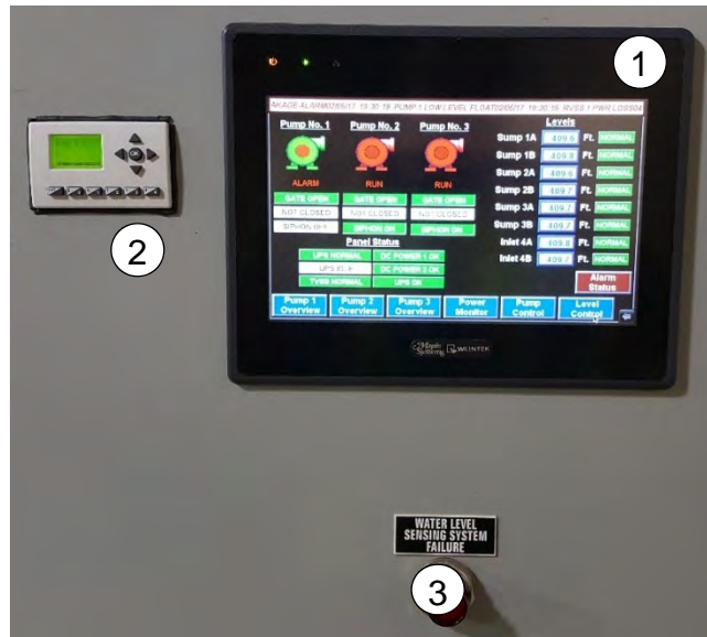
Figure 22.9. Operator Interface Terminal (1) Operator Interface Terminal (2) Monitoring PLC (3) Water Level Sensing Indicating Light
