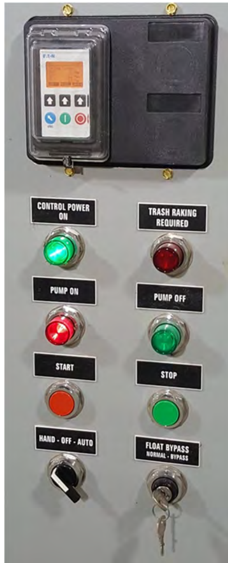
Figure 22.8. Pump Starter Controls
