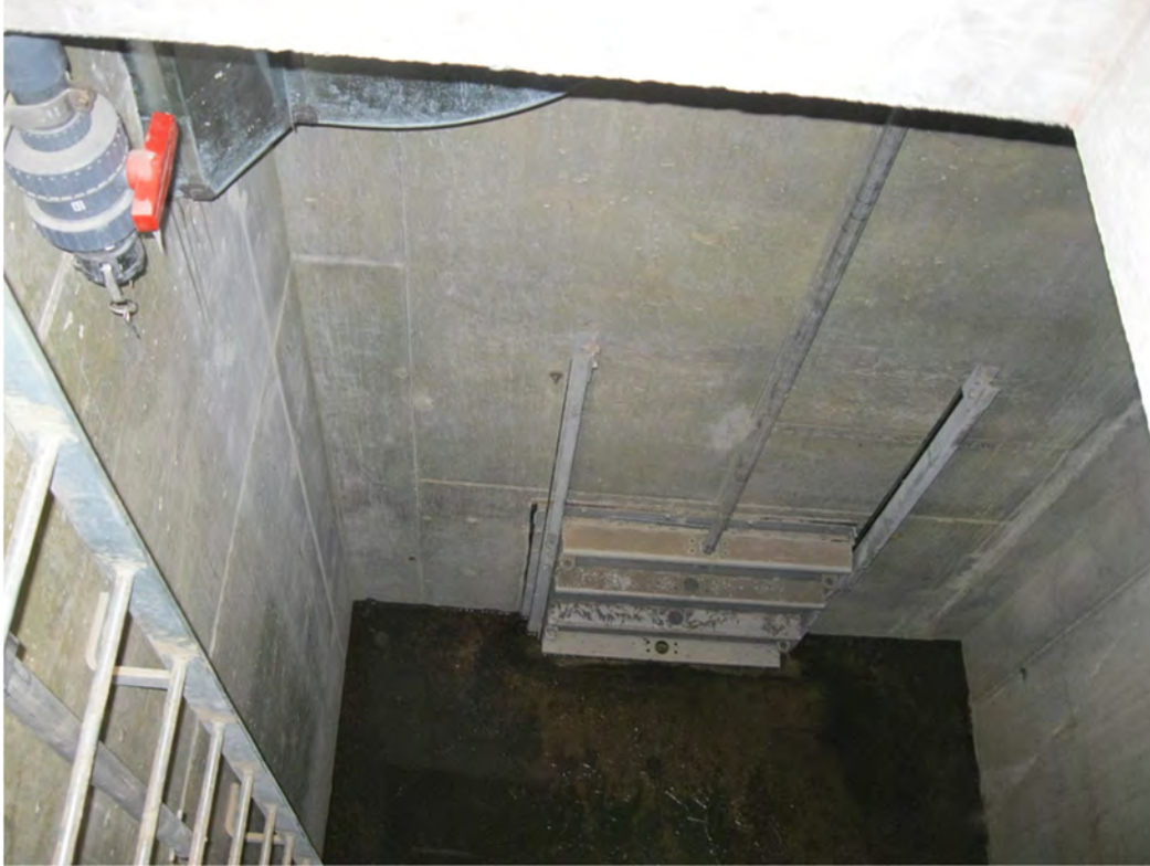
Figure 14.4. Fabricated Stainless Steel Slide Gate
