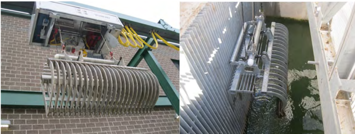
Figure 13.3. Unguided cable trash rake
