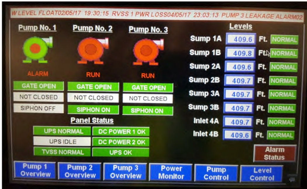
Figure 22.10. Operator Terminal: Pump Station Overview
