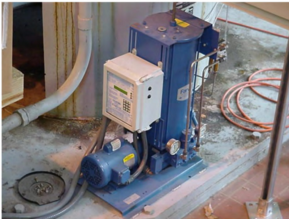
Figure 14.6. Automatic Lubrication System
