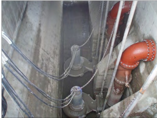
Figure 6.2. Trench well station with submersible pumps in Roseau, MN (courtesy Barr Engineering)
