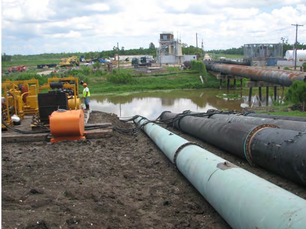
Figure 3.4. Hydraulic driven submersible pumps for temporary pumping
