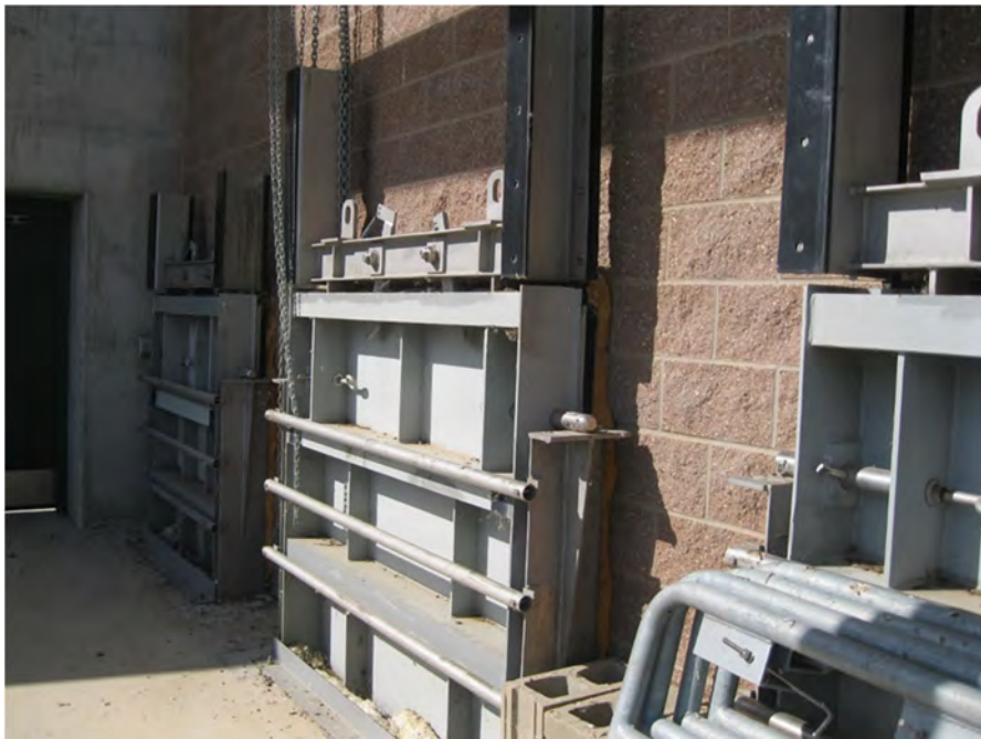
Figure 14.3. Bulkheads placed in front of pump station
