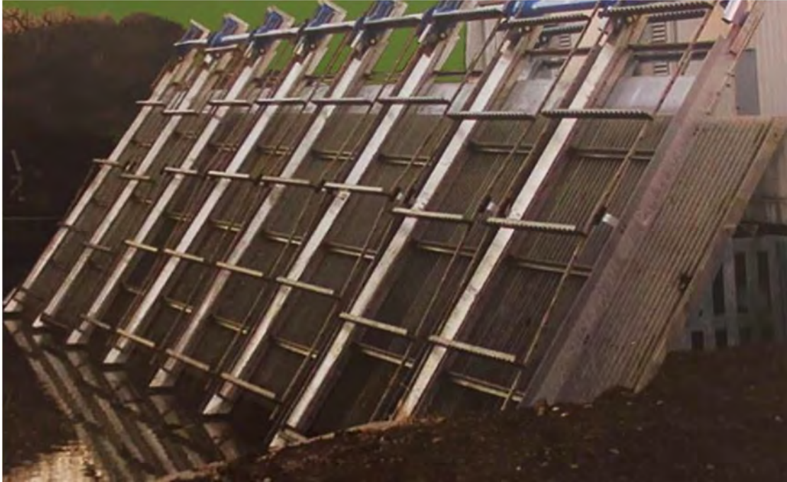
Figure 13.9. Self-Cleaning Trash Rake (outward winding)
