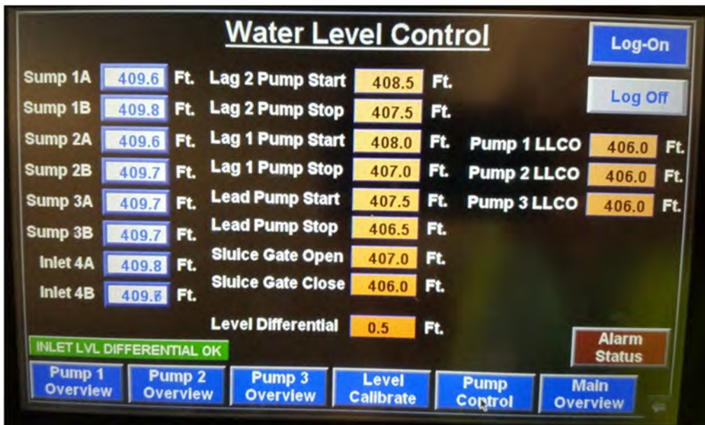
Figure 22.14. Operator Terminal: Pump Start/Stop Elevations
