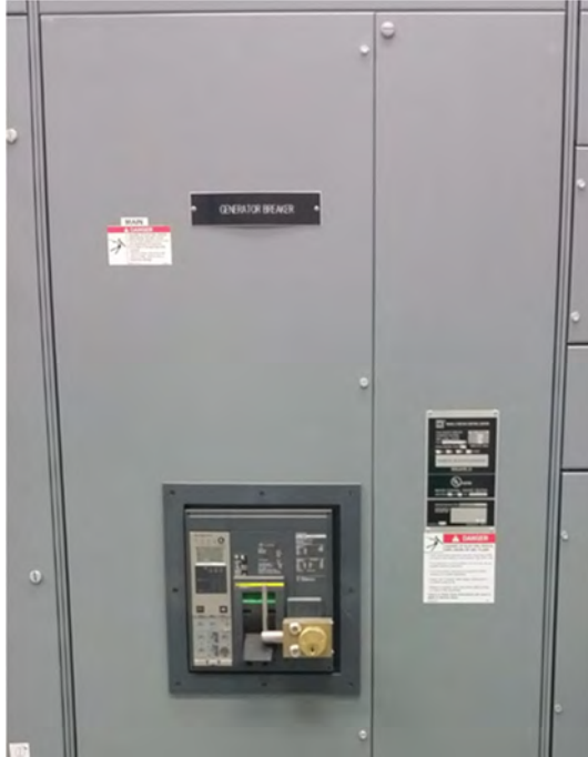
Figure 29.1. Generator Circuit Breaker
