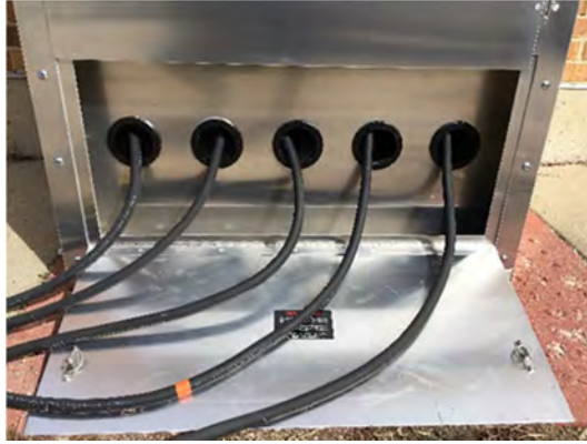
Figure 29.3. Generator Connection Enclosure Field connections
