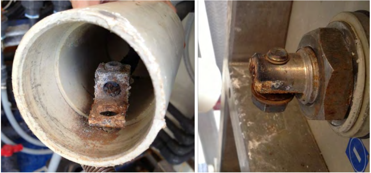
Figure 58.—Damaged EDM cathode electrical connection. Photo taken on 8/29/13,
