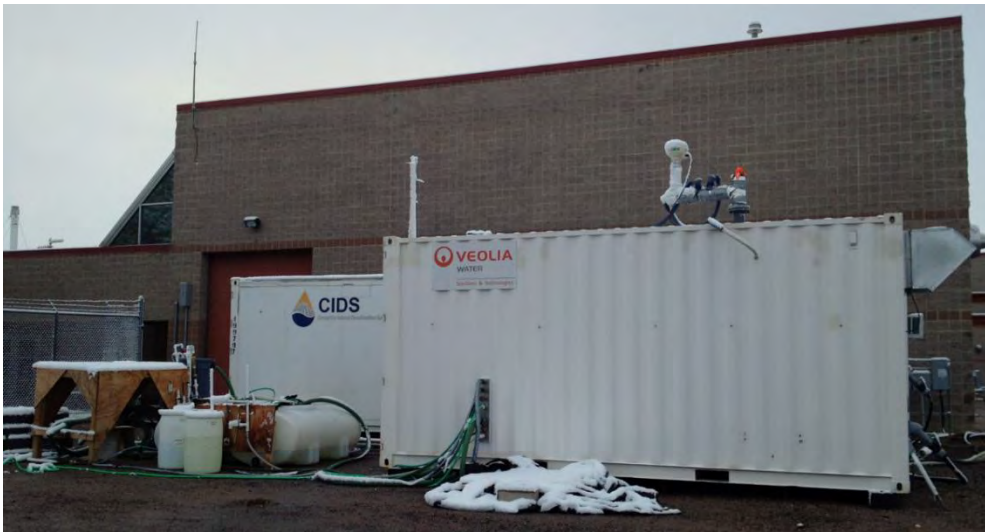
Figure 55.—ZDD system installed in Brighton (20-gpm).
