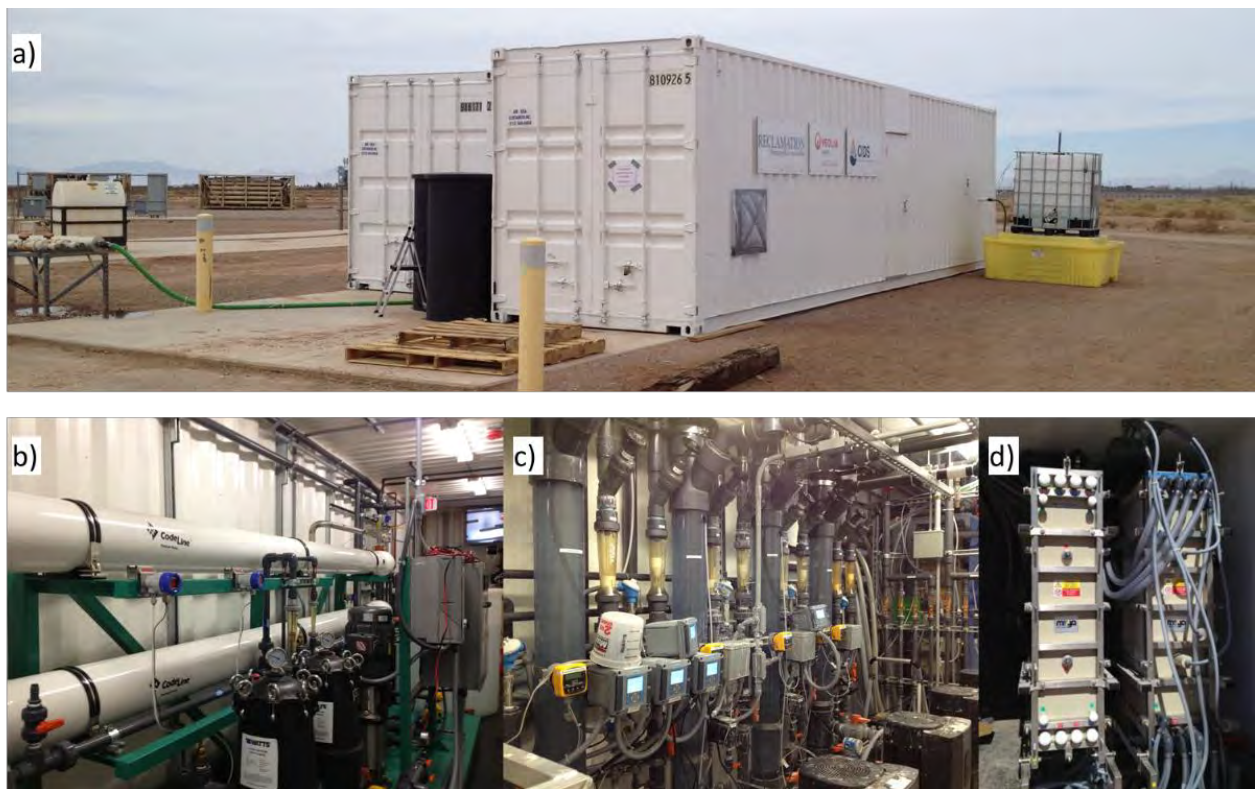
Figure 12.—Phase 2 ZDD System Installed in Alamogordo (40 gpm). Showing a) containers, NaCl tanks, and sulfuric acid tanks; b) NF system; c) EDM standpipes and pumps; and d) EDM stacks.
