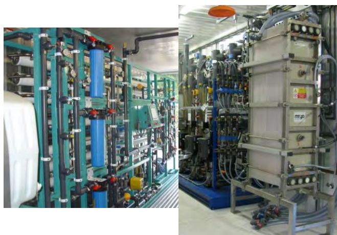
Figure 10.—Phase 1 ZDD system installed in Alamogordo (20 gpm).
