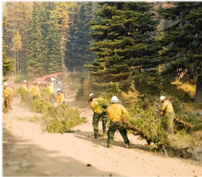
Figure 1. A photo of workers dragging and carrying cut vegetation up a dirt road to a woodchipper.
