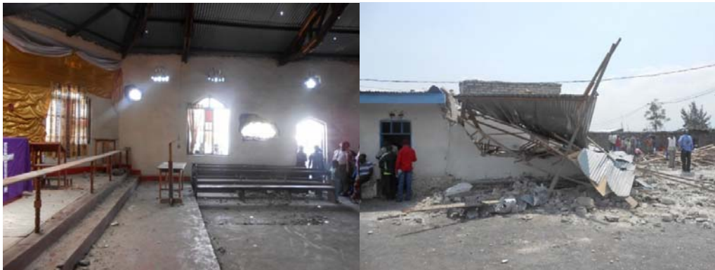
Left: Anglican church. Right: Damaged school.
