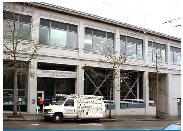
A seismic retrofit of this police station in Seattle, Washington was paid for using capital improvements funds. Structural bracing was added to the building at all levels. The project is highlighted in FEMA's Best Practices Portfolio.
