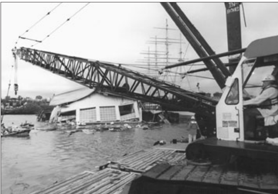
A crane from the Philadelphia District's labor and equipment force removes debris from the Pier 34 site
