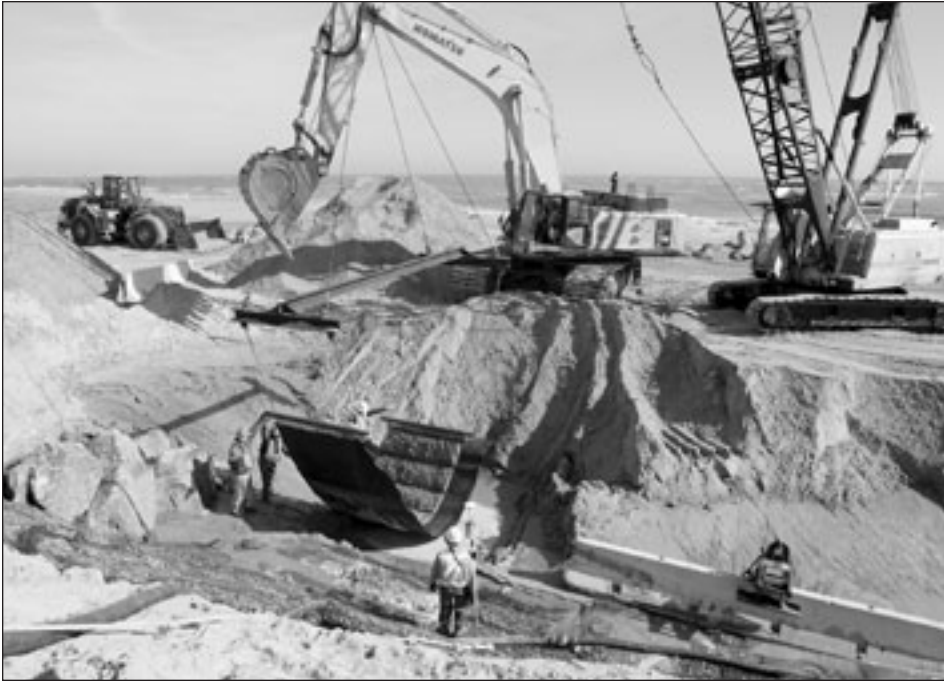
Placement of stone mat foundation for upgrading the Hereford Inlet Seawall, North Wildwood, N.J.
