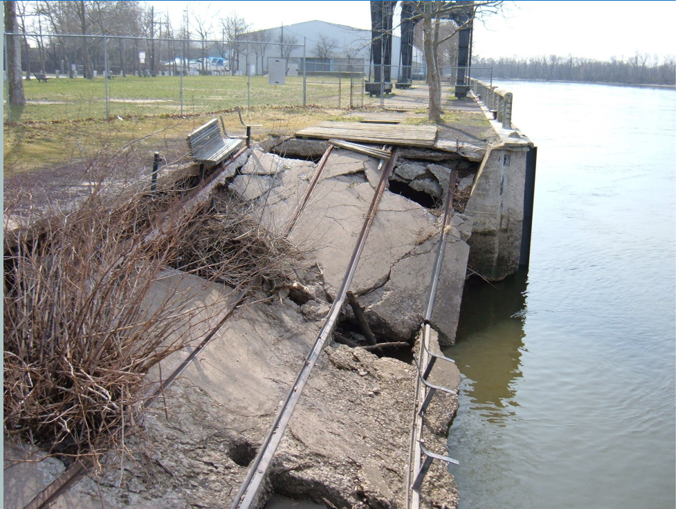
Collapsed section of the pier at the Trenton Marine Terminal
