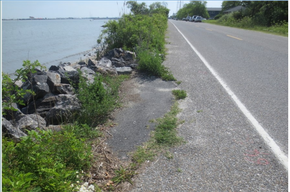
Delaware Avenue in the City of Cape May is threatened by erosive forces from Cape May Harbor.
