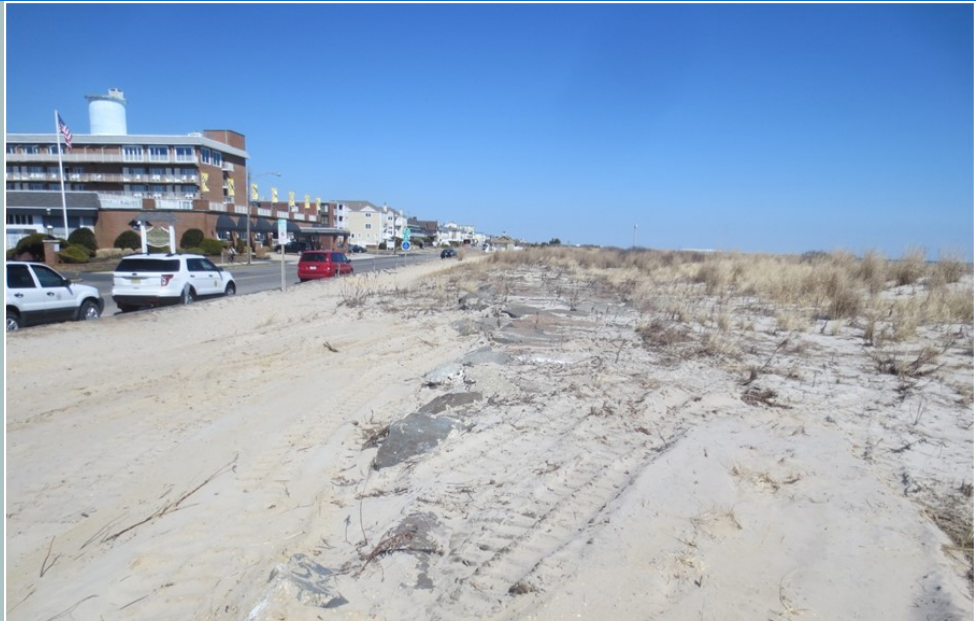
Existing seawall that is located between Beach Avenue and the beach on the south side of the City of Cape May.
