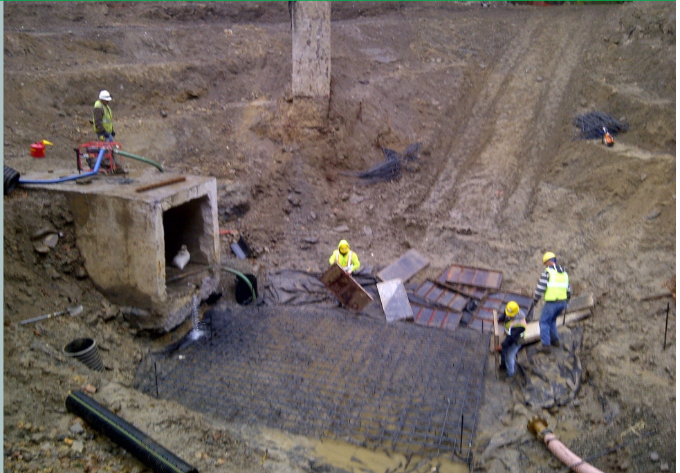
Construction of a vault structure to control sewer overflow along Indian Creek in Philadelphia as part of the Cobbs Creek Habitat Restoration project in 2013.
