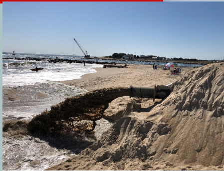
The state of Delaware operates the Indian River Inlet sand bypass plant in Sussex County, DE. Sand is pumped from the south side to the sand-starved north side. Federal construction funds
