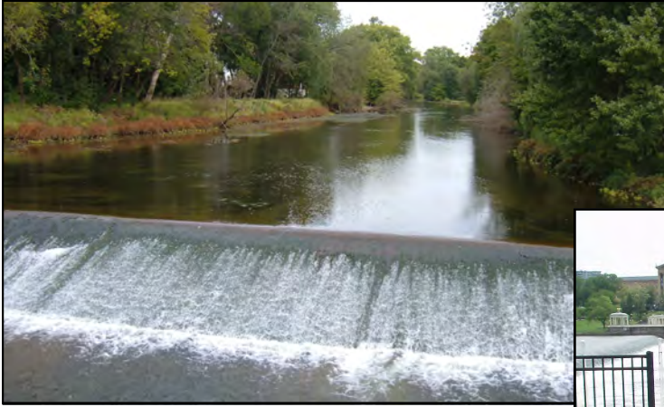
Bloomsbury Dam on Musconetcong River, NJ: The project involves the removal of the dam to enhance aquatic habitat and to restore the connectivity of 8 miles of a Federally-designated National Wild and Scenic River.
