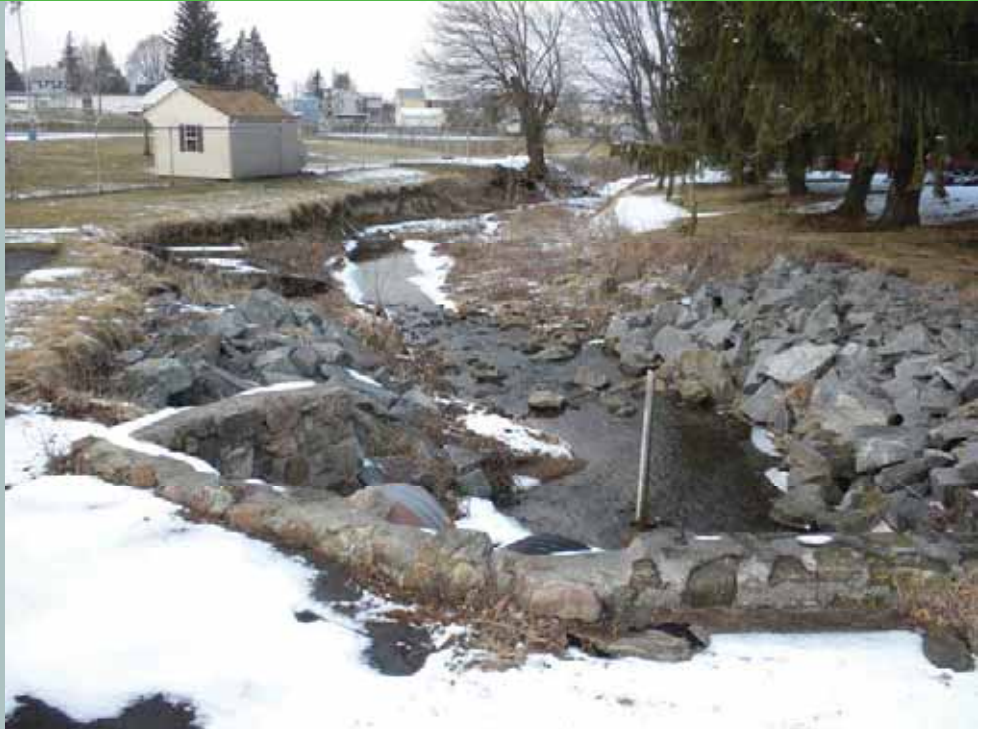
Flows under State Route 1010 (Weiss Street) from Toad Creek are continually eroding Tipton Borough's municipal recreation facility property.
