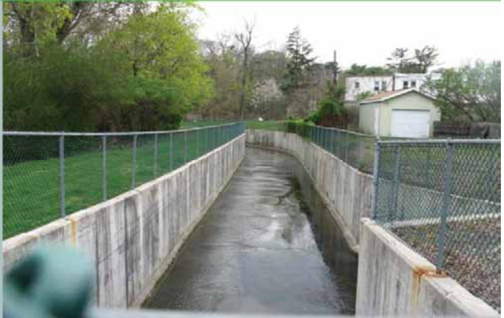
Portions of the creek are channelized in concrete flumes. This might appear to help the problem in one area, but only pushes the flooding problems downstream.
