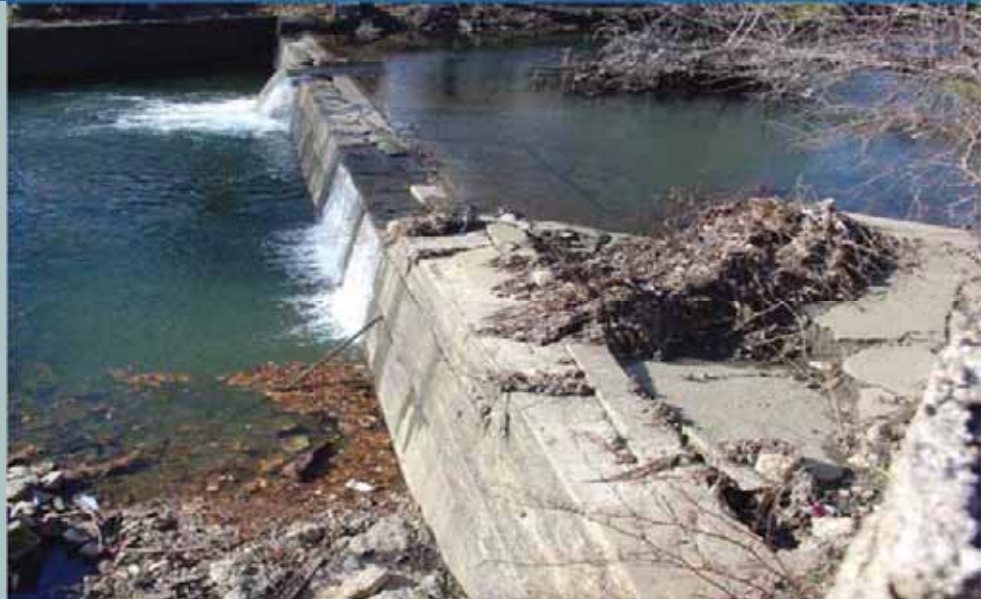
The Woodland Avenue Dam is the first impediment along Cobbs Creek preventing fish passage. Stored sediment behind the dam must be controlled during removal to prevent adverse upstream impacts.
