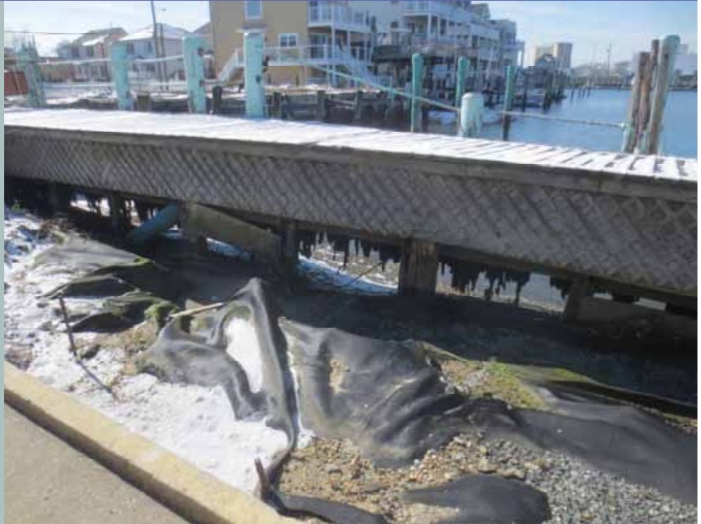
The photo above shows the deteriorated condition of the Bulkhead at Massachusetts Avenue in Atlantic City.
