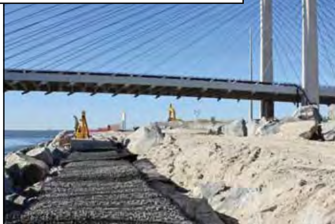
Indian River Inlet, DE: Post-Sandy work to reinforce the north jetty involved placing marine mattresses, filling voids and positioning capstones.
