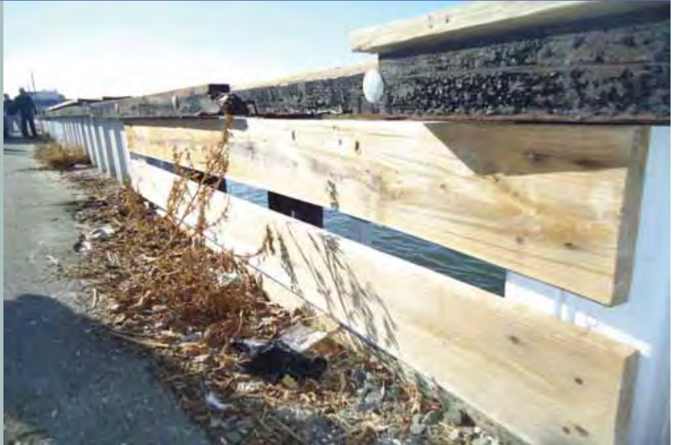
This photo shows the poor condition of the bulkhead in Ventnor that leaves property and infrastructure vulnerable to storm damages.
