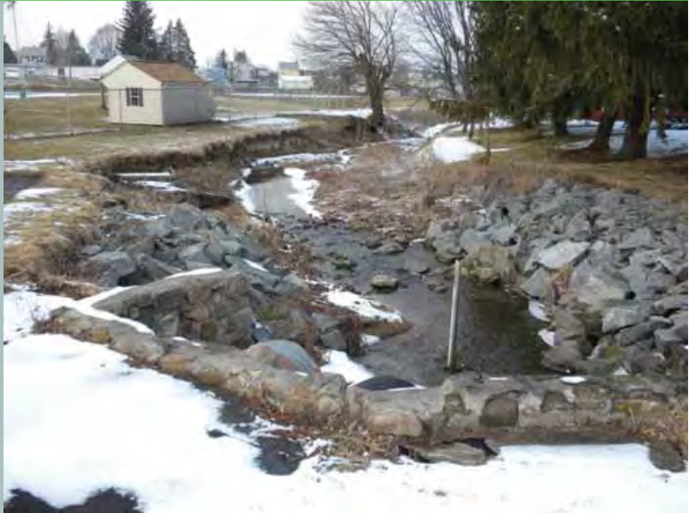
Flows under State Route 1010 (Weiss Street) from Toad Creek are continually eroding Tipton Borough's municipal recreation facility property.
