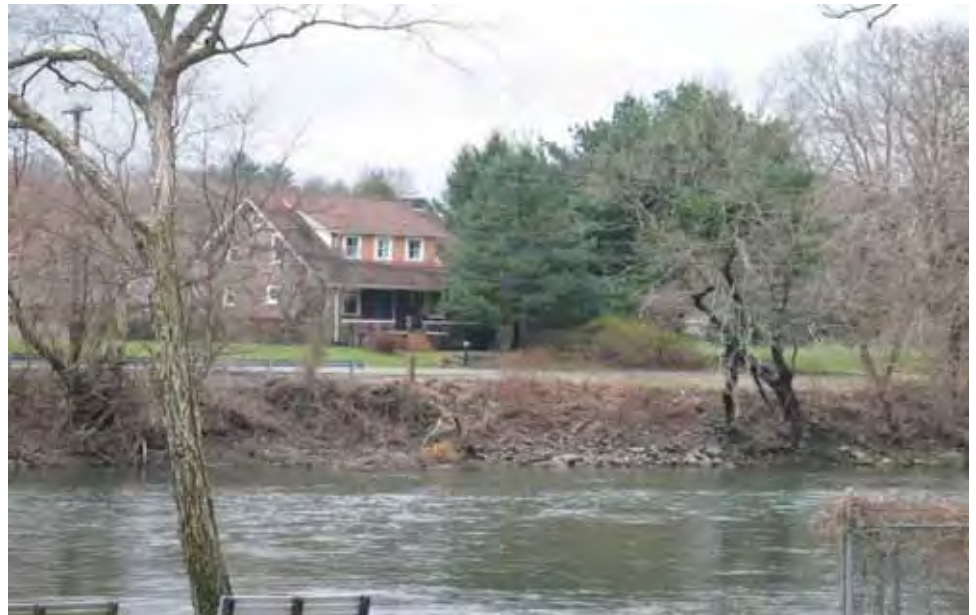
Erosion of the right bank of the Schuylkill River along River Road in North Coventry Township, PA.
