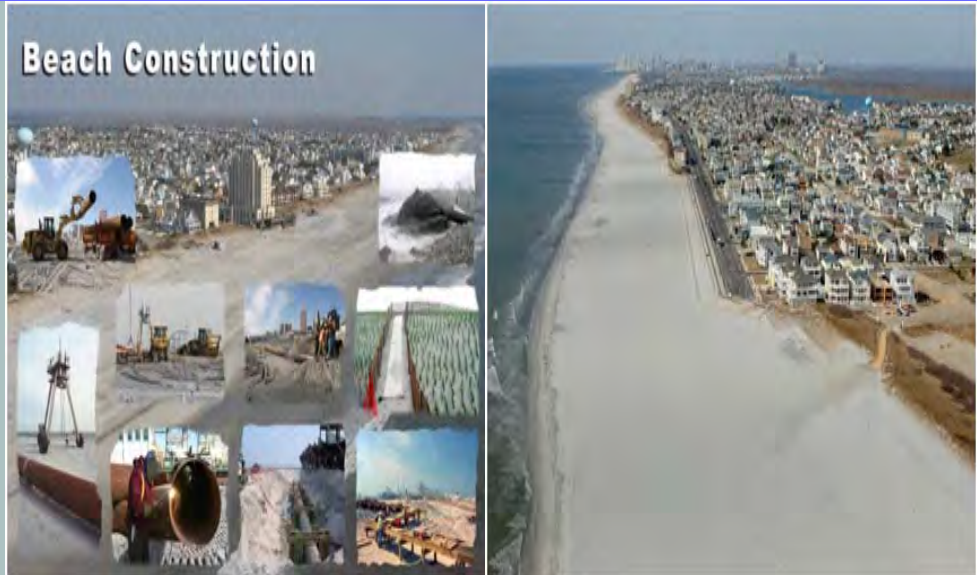
Left: Initial Storm Damage Reduction Beach Construction - Brigantine Island. Right: Aerial Photo of the Completed Storm Damage Reduction Beach fill – Brigantine Island.
