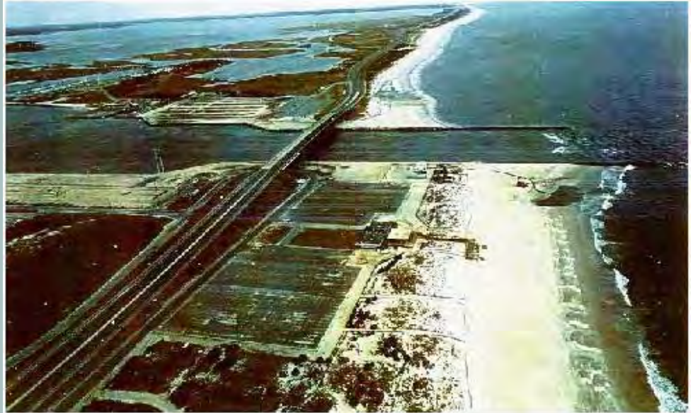
Indian River Inlet, Delaware, looking to the north showing the portable sand bypass system excavating a hole in the south fillet at the inlet. The system consists of a crane that holds an educator pump that removes sand from the beach face, two pumps to move the sand over the bridge, and a discharge line on the north side that discharges the sand onto the beach (where it looks wet in the photo).
