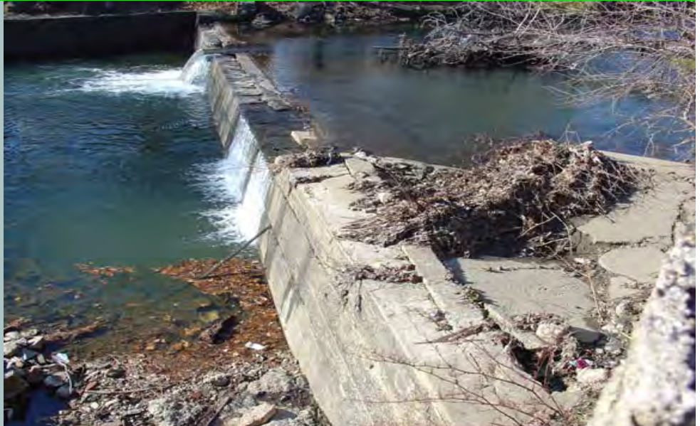
The Woodland Avenue Dam is the first impediment along Cobbs Creek preventing fish passage. Stored sediment behind the dam must be controlled during removal to prevent adverse upstream impacts.
