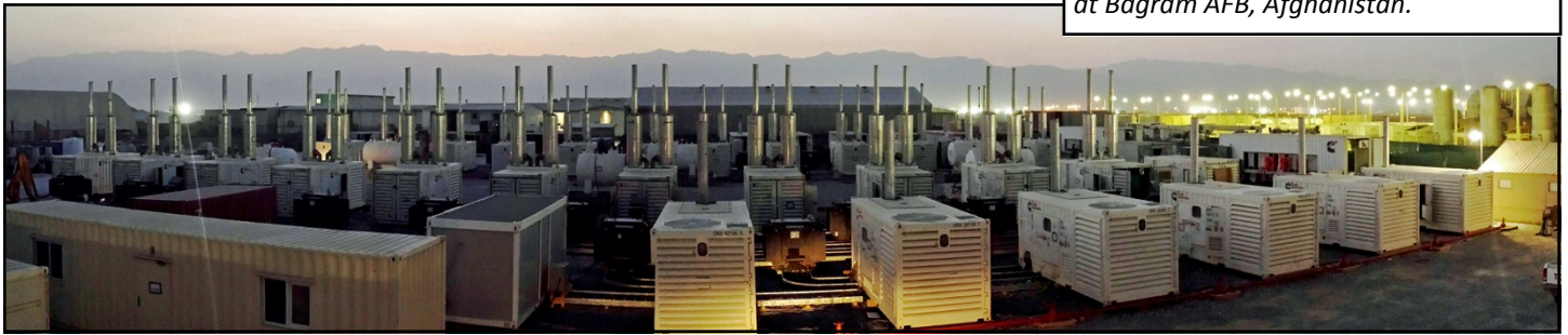
Global Power Program: Managing more than $1 billion in contracts to date, the District works with the Army's 249th Engineer Battalion on projects such as this temporary 30-megawatt installation at Bagram AFB, Afghanistan.
