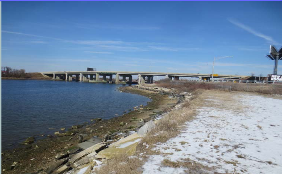
The area near sunset avenue in Atlantic City is protected by a low poorly constructed rubble revetment that is easily overtopped by storm surge during flood events
