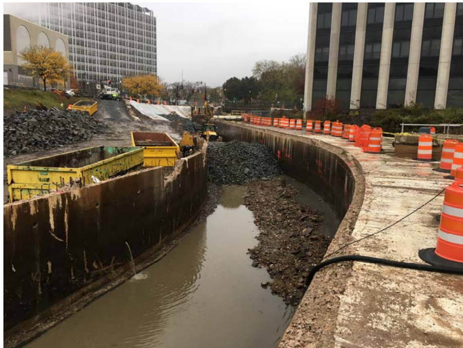
Downstream view of demolition of the existing culvert along Assunpink Creek in downtown Trenton, NJ
