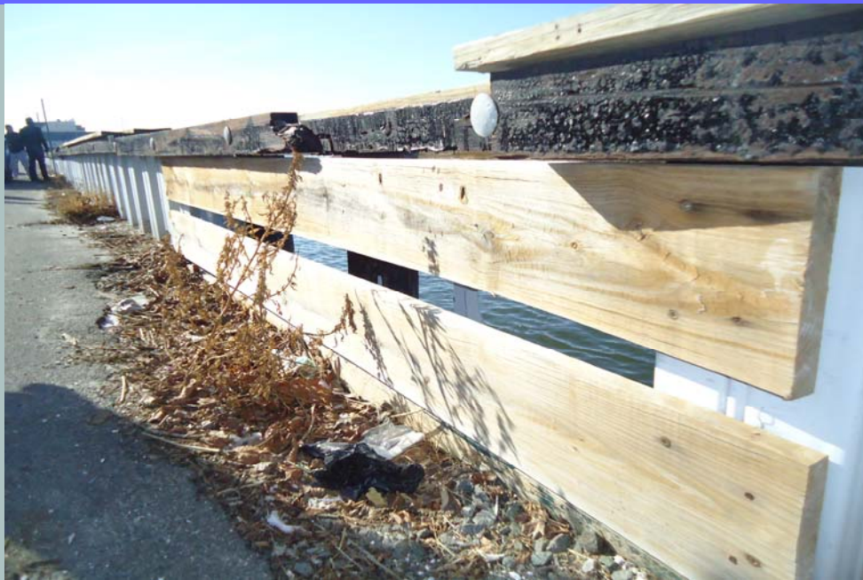
This photo shows the poor condition of the bulkhead in Ventnor that leaves property and infrastructure vulnerable to storm damages.
