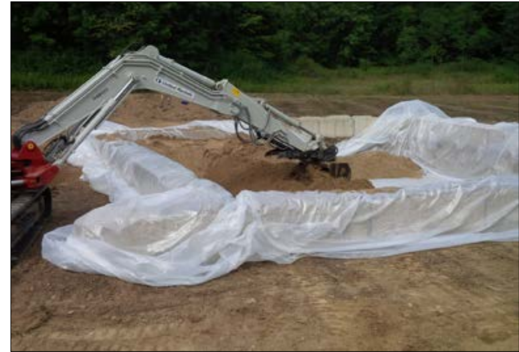
(Photos by John Day) Sand being placed into the base of the Permanent BEM at Camp Ravenna, Ohio.
