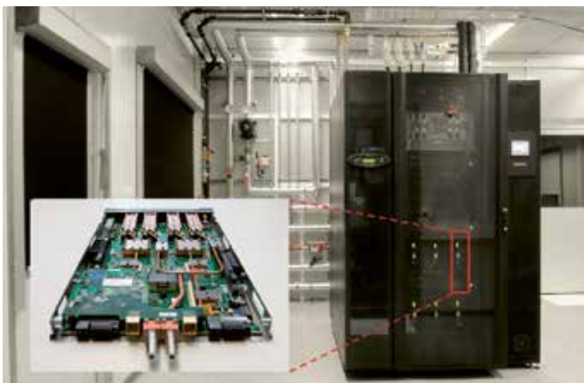
Figure 2: AQUASAR; the detail shows a typical board with water cooled chip structures
