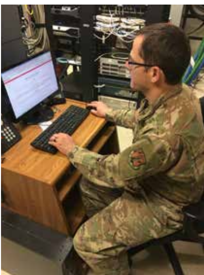
Master Sgt. Samuel Blunck configures phone systems in the switch room at the Rolland R. Wright Air National Guard Base, Utah, Aug. 15, 2019.
