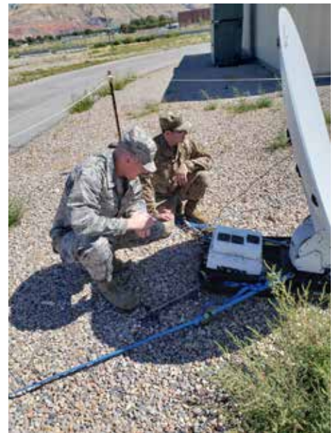
Master Sgt. Sam Blunck and 1st Lt. Tyler Olsen set up the satellite dish for the Joint Incident Site Communications Capability Sept. 15, 2019.
