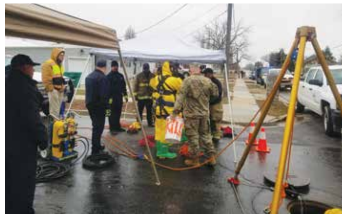
After Layton City residents noticed a gas smell in their homes and water, the 85th CST made a confined-space entry using self-contained breathing apparatus on two Soldiers to take water and air samples. This critical assistance used highly trained National Guardsmen with sophisticated equipment unavailable to the city of Layton.
