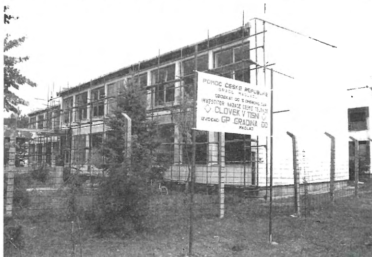
Maglaj primary school reconstruction project. All work was completed during the summer vacation period to avoid disruption of the regular class schedule.
