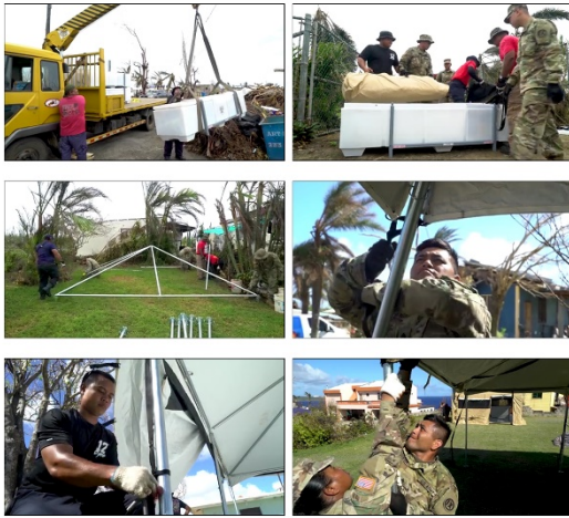
U.S. Soldiers with the 797th Engineer Company, Army Reserve, and members of the Commonwealth of Northern Marianas Islands Department of Fire and Emergency Services build tents for homeowners after Super Typhoon Yutu destroyed their homes Nov. 13, 2018 on Saipan, Commonwealth of Northern Marianas Islands. Teamwork and communication between the services and the CNMI Fire Department were instrumental in relief efforts after Yutu. (U.S. Air Force video by Staff Sgt. Bethany La Ville)
