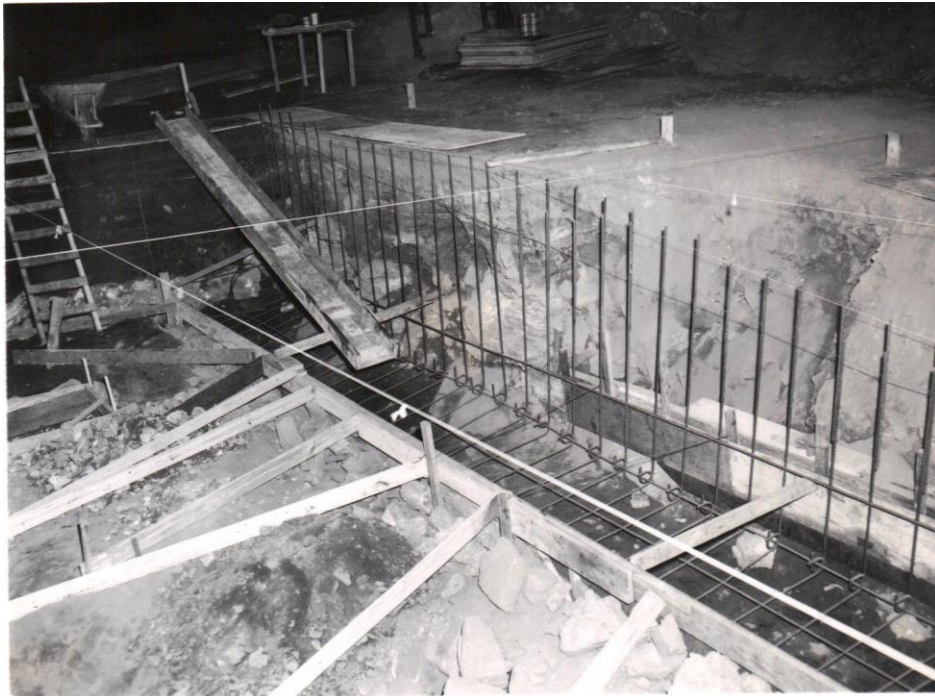
Figure 7. Reinforcing steel (rebar) was put in place to secure the retaining walls (9/14/64).
