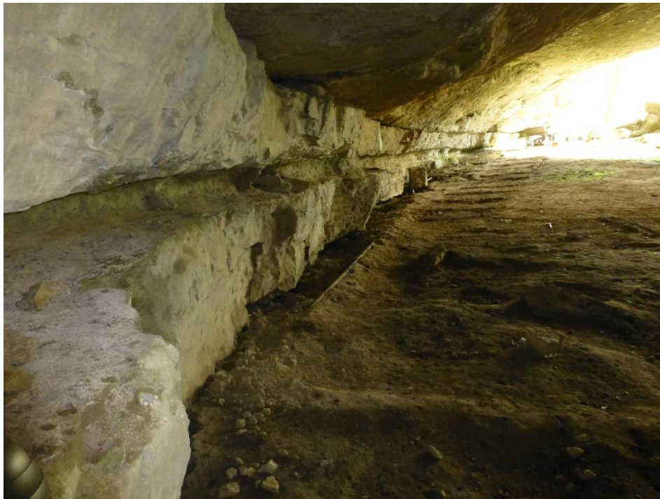
Figure 18. Current (2016) area along northwest cave wall showing scalloping, erosion, exposed conduit, subsidence, and slumping. Ground disturbance from previous walkway and exhibition constructs is also present.
