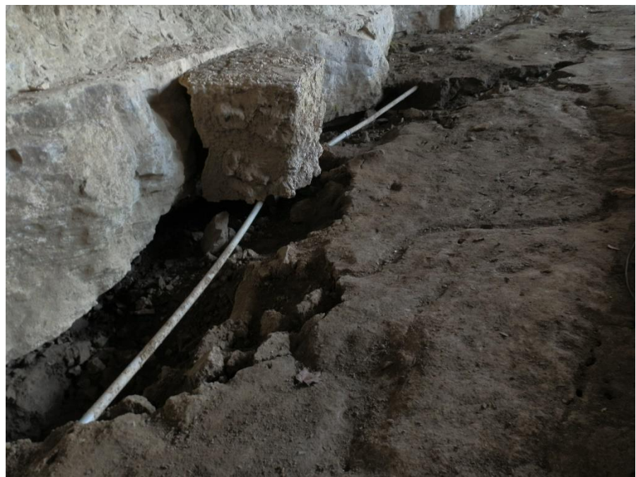
Figure 17. Soil loss along north wall (Seibert 2010). Photos courtesy NPS SEAC.
