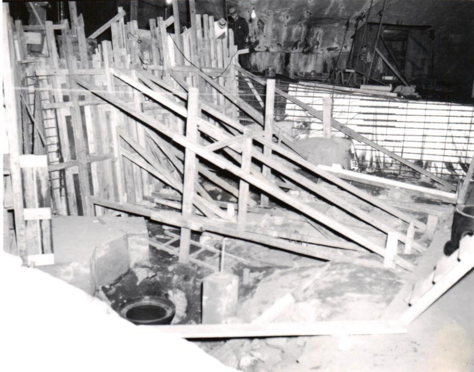
Figure 8. Construction for a viewing platform to allow visitors to see the cave stratigraphy. (Photo courtesy NPS, RUCA 10/16/64).
