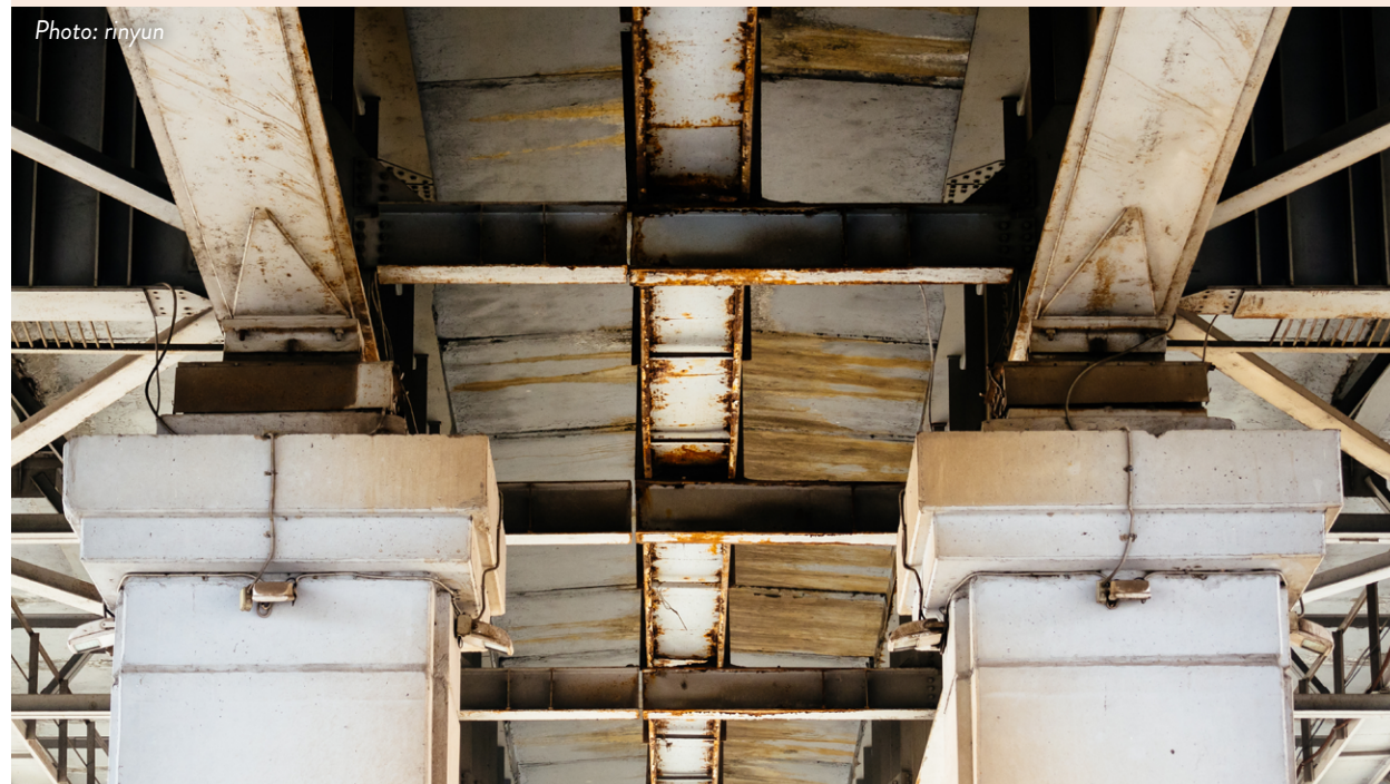
CONCRETE COLUMNS AND RUSTY METAL OF THE OLD BRIDGE.
