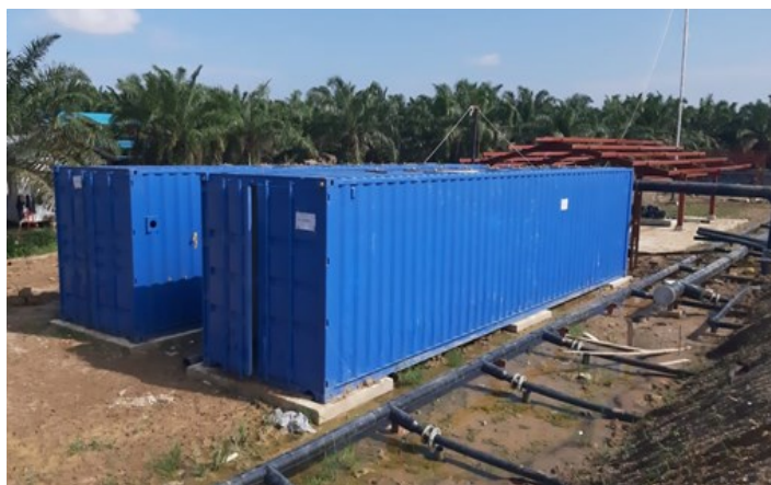
Image: Elmoz biogas biological scrubber installed at PT. Pasadena Biofuel Mandiri (Source–PT. Elmoz GEO Solusi).
