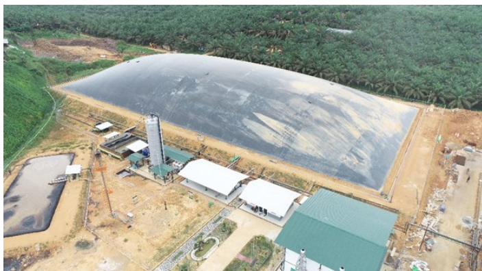
Image: Biogas power plant at PT. Swadaya Multi Prakarsa (Source-PT. Elmoz GE Solusi).
