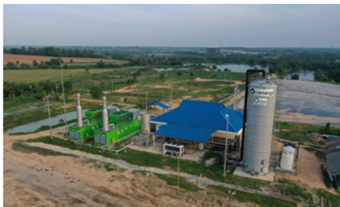
Image: Hampan biogas power plant (Source-PT. GREE Services Indonesia).
