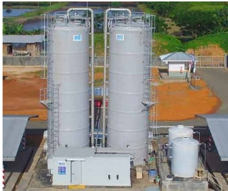
Image: Biogas column scrubber (Source—biogasclean.com).
