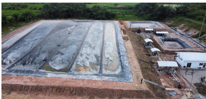
Image: PTPN V biogas co-firing boiler plant under construction (Source-PT. Ecody Agro Energi).
