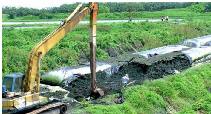
Image: POME sludge captured by TenCate Geotube® Dewatering (Source-TenCate Geosynthetics).
