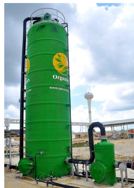
Image: Organics Bali bio-scrubber installation (Source–PT. Organics Bali).
