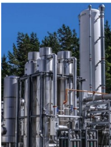
Image: CarboTech biogas upgrading plant in Sofielund, Sweden (Source–Carbotech).
