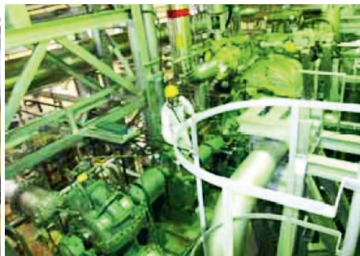
HPCI (Unit 5 side, with light)
