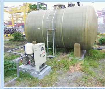
Wasted water recycled system
