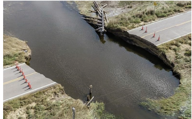
A bridge on 406 th Avenue in Davison County was completely washed away by flooding.
