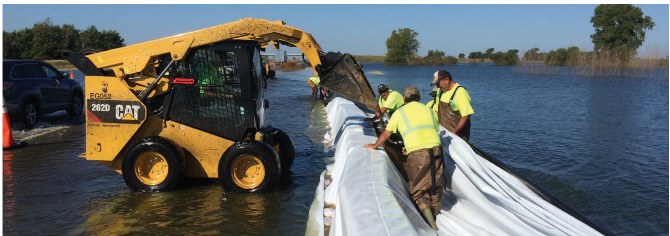
Maintenance crews install a temporary barrier to hold back flood waters on I-90 near Bridgewater, SD.
