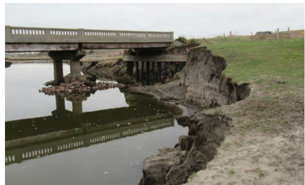
Embankment washout on 272 nd Street in Hutchinson County.
