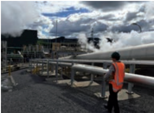
Geothermal Power Plant in New Zealand
