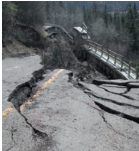
Road in Edmonton destroyed by a landslide
