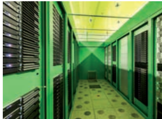
High Performance Computer facility at ETH.
