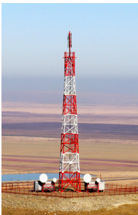
One of Russia's 4900 Transmission Stations
