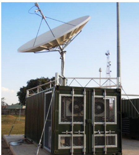
DVB-T2 transmitter site – Lukasa, Zambia (Photo: Steven Vorster)
