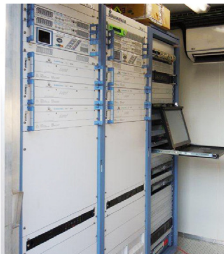
DVB-T2 transmitter installation (Photo: Steven Vorster)
