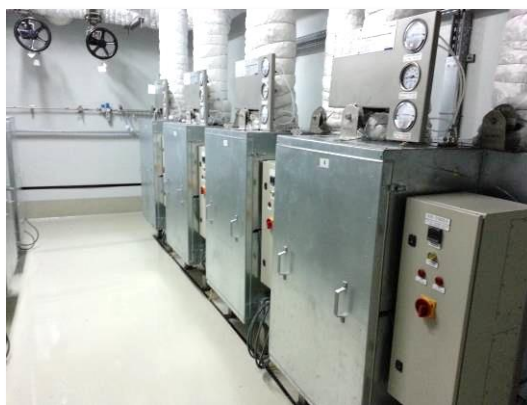
Figure 7.12. One of the two groups of high-efficiency particulate air filters
