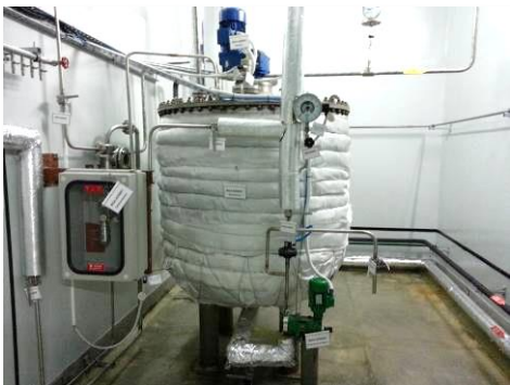
Figure 7.10. LRW: The warmed tank with mixer for contaminated oil
