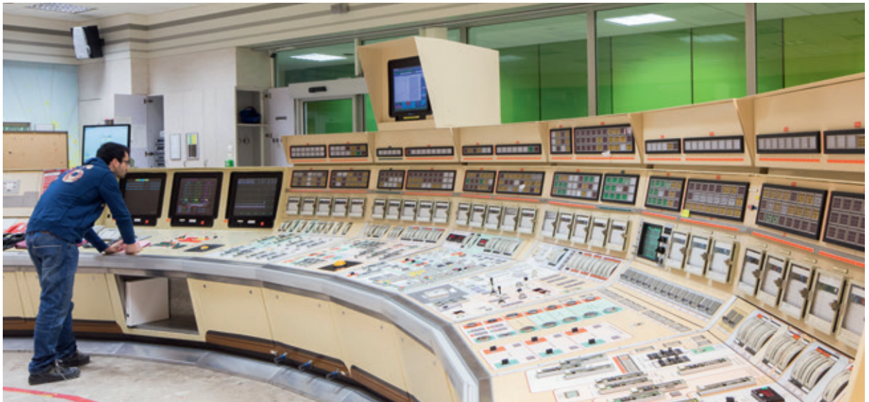
Control room. EDF, France
