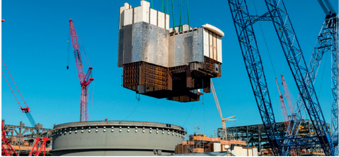
Vogtle Unit 4 - AP1000, United States, August 2016 CA20 module placed. Georgia Power Company
