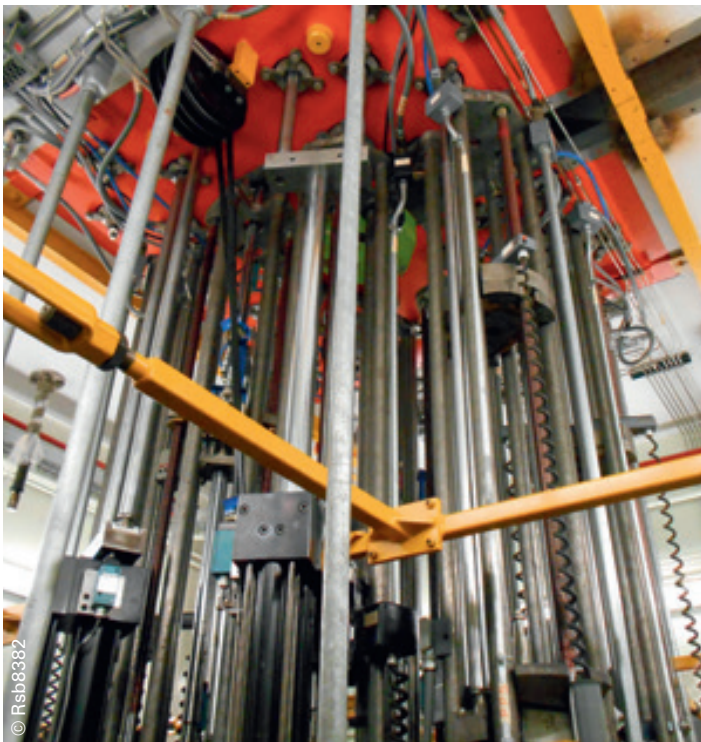
TREAT subpile room, Idaho, United States.
