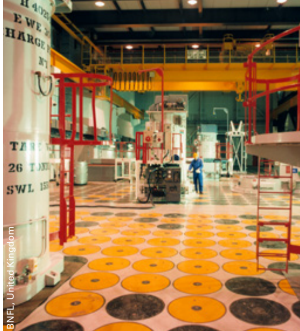
View of a vitrified waste product store.
