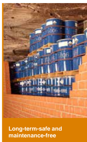
Figure 8: Installation at UTD Herfa-Neurode
