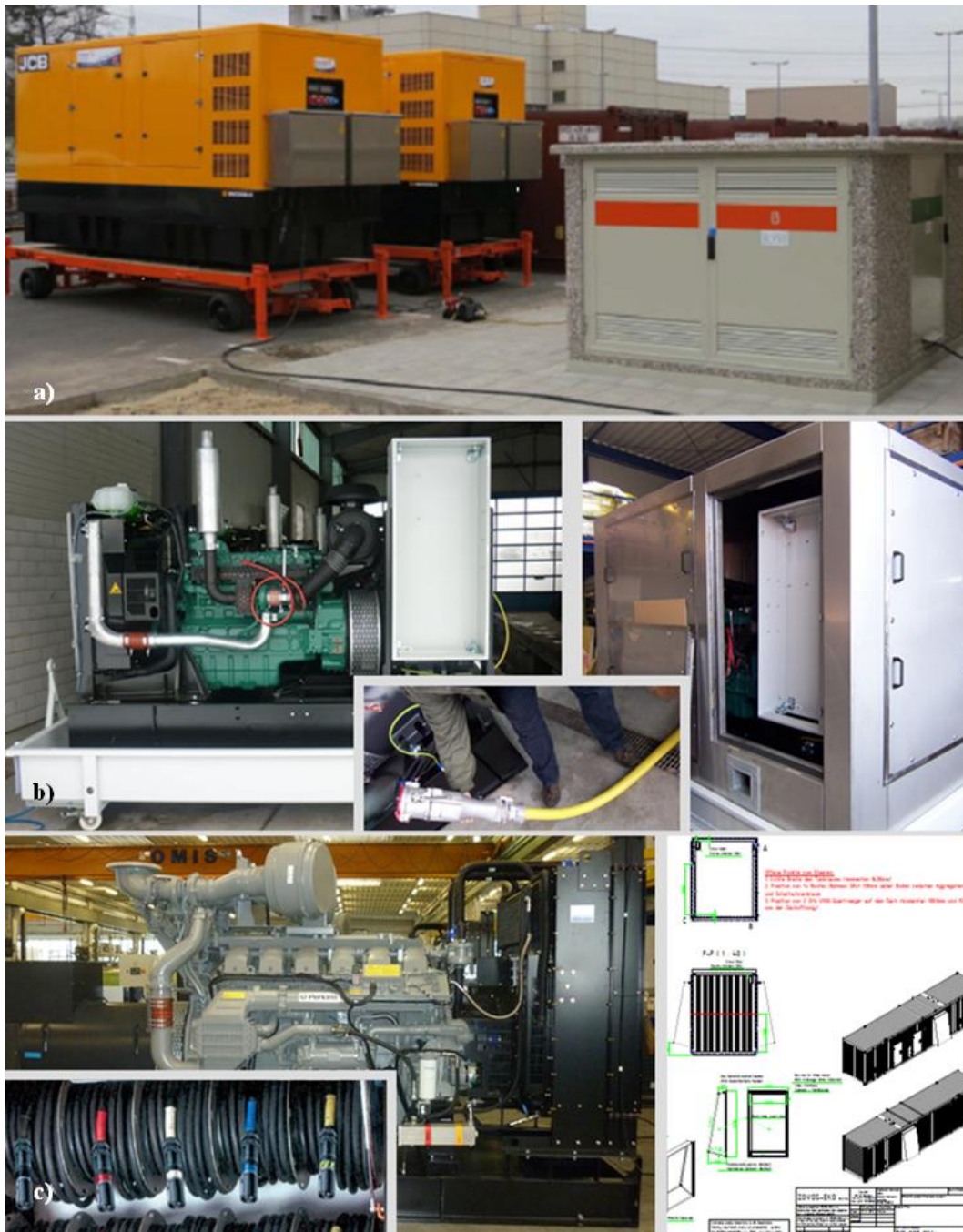
Figure 3: a) Two medium sized (550 kVA) mobile EDG in trailer-container; feeding point. (Source: RWE). b) Small sized (200 kVA) mobile EDG that can be handled without machinery; connector cable and housing. c) Big sized (1250 kVA) mobile EDG; multiple connector cables for manual manageability; trailer-container for big sized EDG. (Source b) and c) : e.on)
