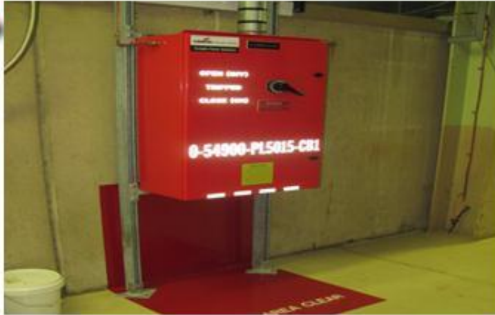
Panel for 400kW AC generators
