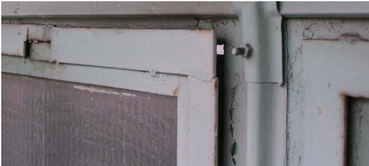
Figure 4. Leakages of the windows “VEKA”, no sealing installed
