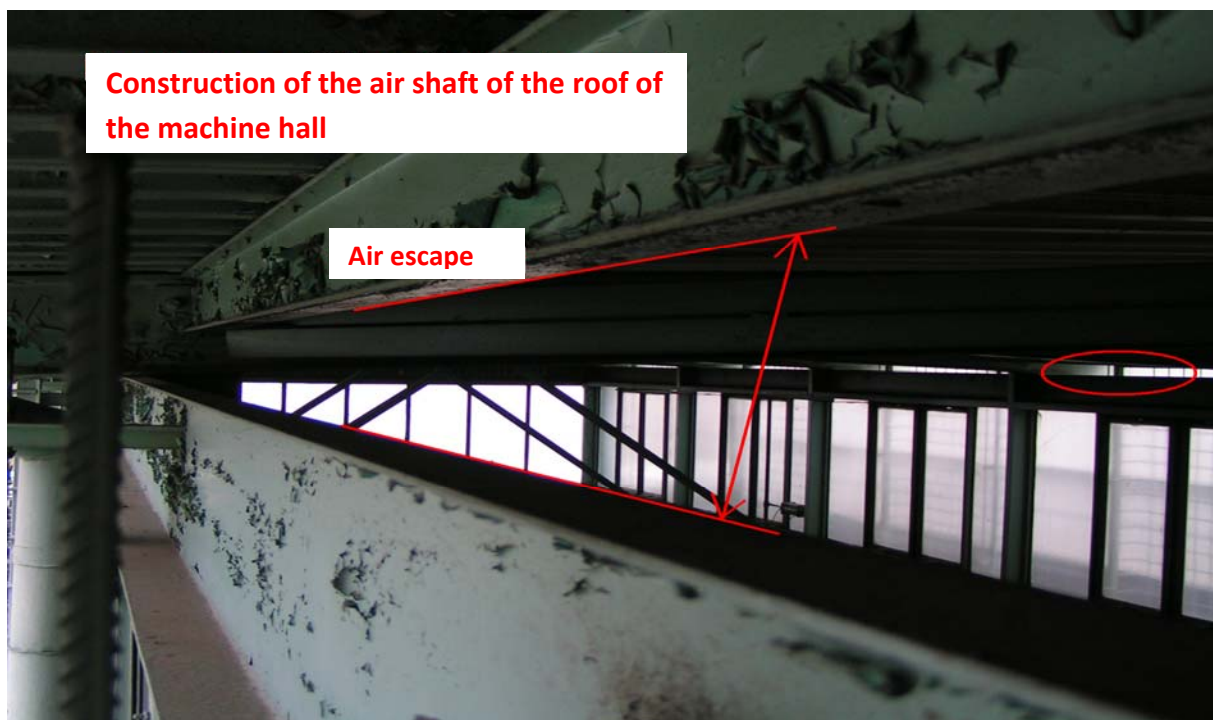
Figure 5. Air escape in the roof construction (marked with the ellipse)
