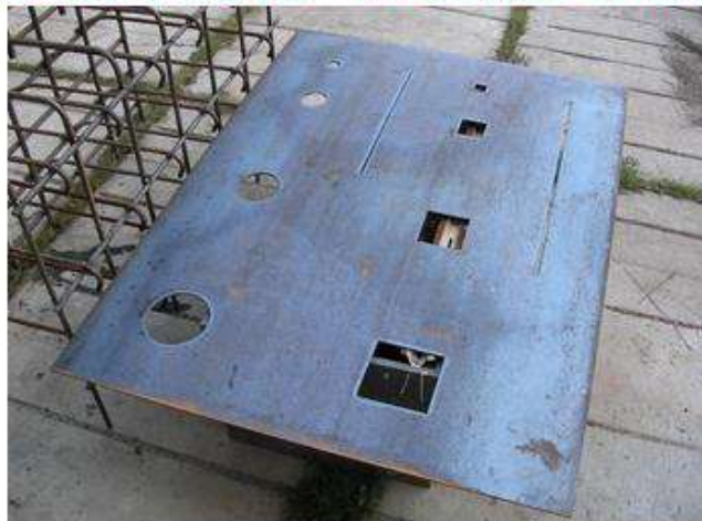
INTERNAL LINER WITH DEFECTS
