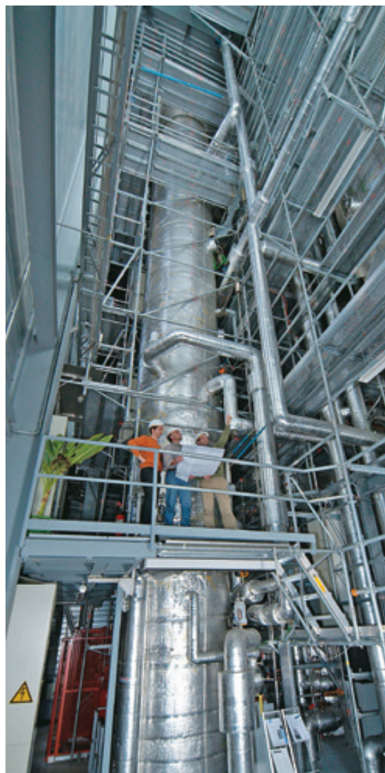
The PANDA reactor pressure vessel. Paul Scherrer Institute, Switzerland
