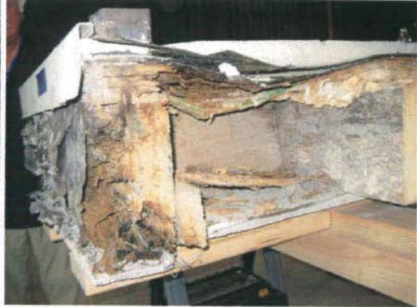
Unit 305 Balcony Remnant Photo 6070 – 6 October 2015
