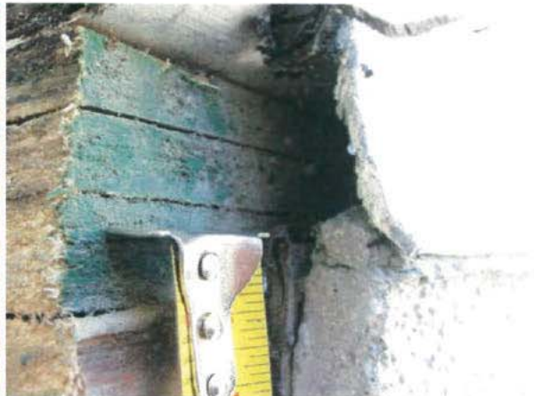
Unit 305 Balcony Remnants Photo 5710 – 29 July 2015
