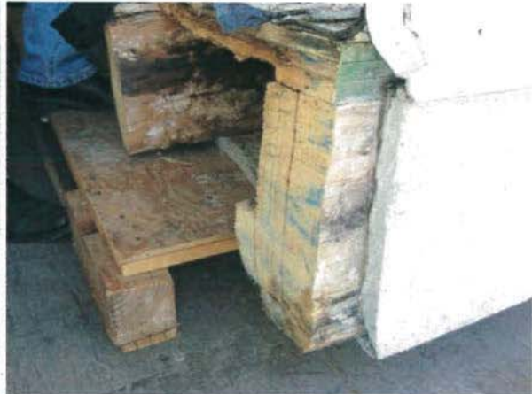
Unit 305 Balcony Remnants Photo 5703 – 29 July 2015
