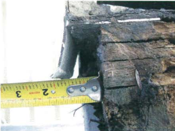
Unit 305 Balcony Remnants Photo 5646 – 29 July 2015
