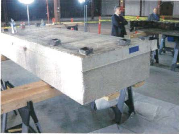
Unit 305 Balcony Remnant Photo 6062 – 6 October 2015
